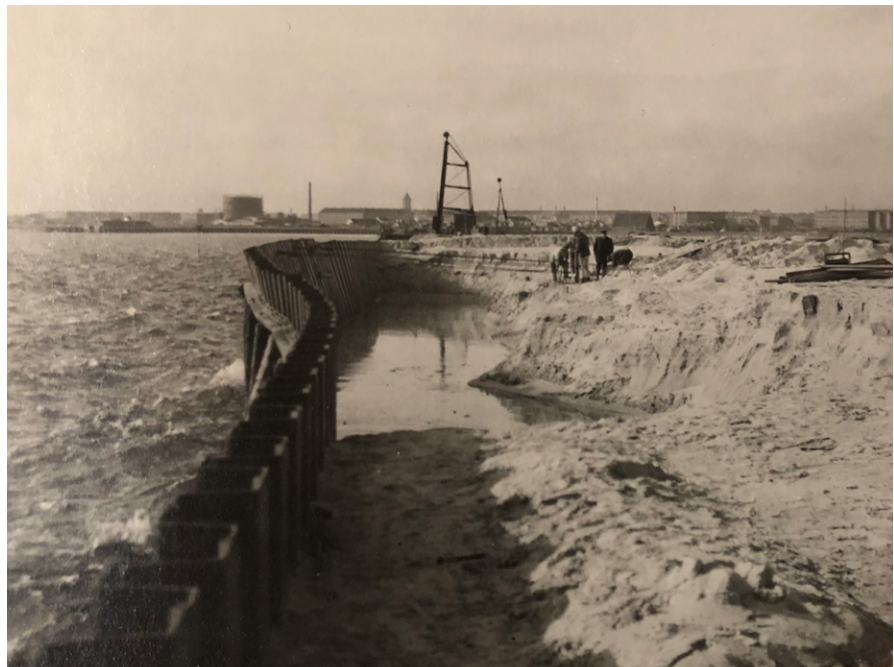
Fig. 1.12 Soil infill process. Archival photograph of the construction of Petrol Island, 1930's, from the By og Havn archives.
