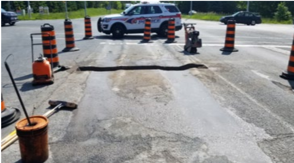
Figure 2-2: Rutting in Approach Intersection at Heavy Truck Traffic Road in York Region 2018
