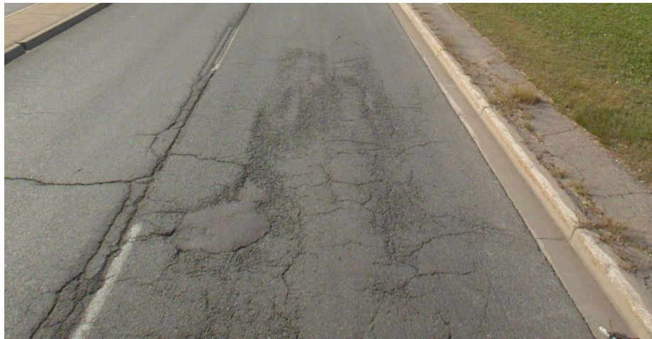
Figure 2-8: Fatigue (Alligator) Cracking – York Region 2018
