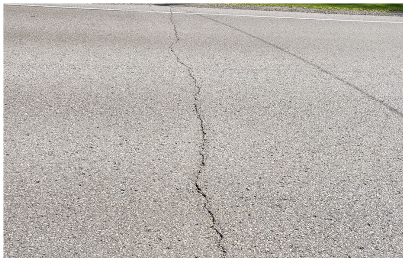
Figure 2-9: Low-Temperature Cracking - York Region 2018
