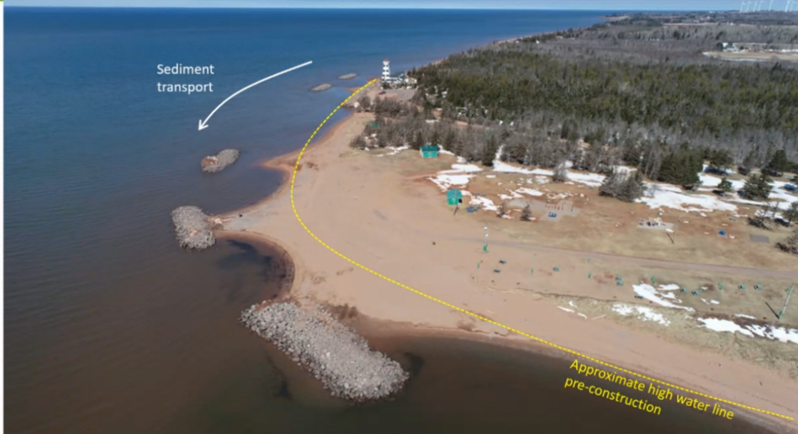
Figure 3.13 Photo illustrating the impact the reefs have on restoring the shoreline at West Point Lighthouse, West Point, PEI. 2022. Image by CBCL.
