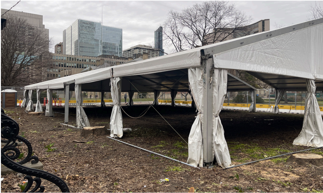
fig. 6.5 At the corner of the Osgoode Hall courtyard, Metrolinx is planning the construction of a subway entrance for the Ontario Line. Metrolinx began axing the trees without public consultation. Many community members were devastated by the loss of some of the oldest urban trees left in downtown Toronto.
