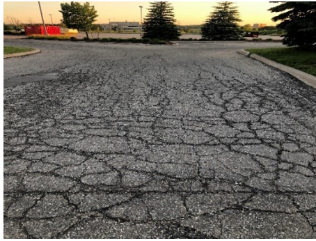
Figure 1-13 Fatigued cracking in pavement (Waterloo, Canada)
