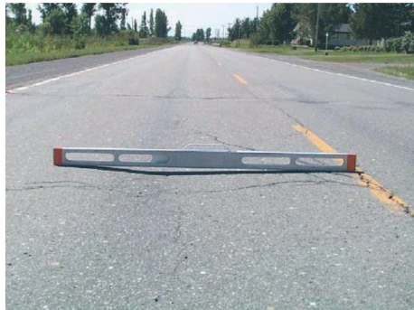
Figure 1-12 Permanent deformation damage [58]
