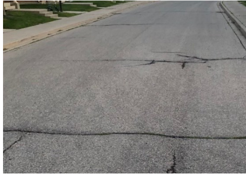
Figure 1-15 Low-temperature (transverse) cracking (Waterloo, Canada)
