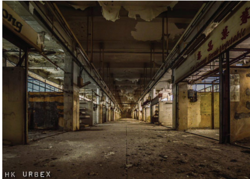
Fig.5.03 Central Market was left abandoned in 2003, leaving the building vacant and exposed to natural elements causing extreme damage especially to structural systems.
