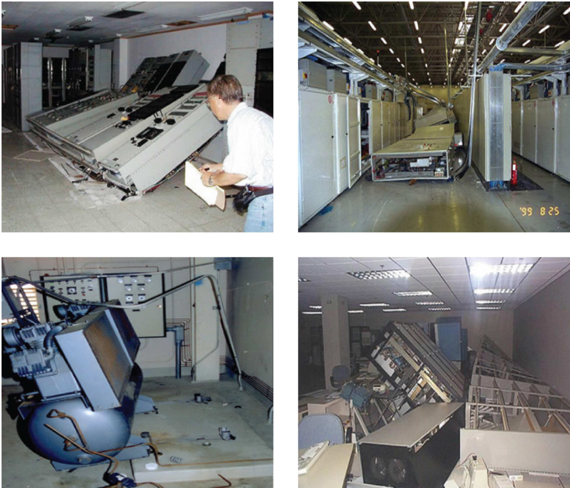
Figure 1.1 Damage of secondary system in earthquake events.
