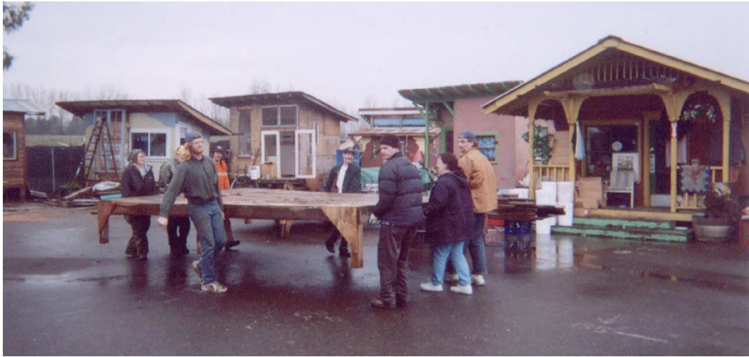
Fig. 26. This photo's caption in the Dignity Village online archive is: "Villagers siting the deck for a house". The community was sanctioned in 2004. (Photo retrieved from https://dignityvillage.org/history/photos/ ).
