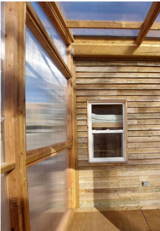
Fig. 111. The v1 polycarbonate panels could be adapted to a smash-resistant clerestory window. (Photo by author).
