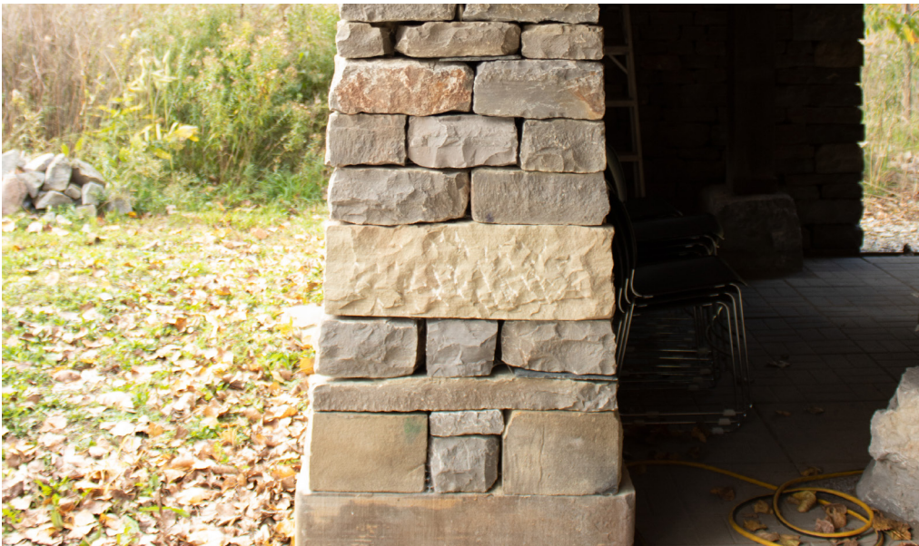
Fig. 2.12 Sample Dry-stone stacked wall at Willowbank, showing variation in stacking pattern, image by author.
