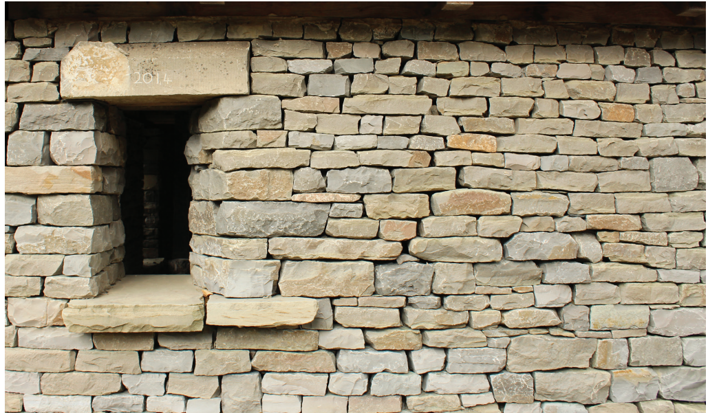
Fig. 2.15 Dry-stone stacked pavilion at Willowbank, showing a mix of colour and texture in stone walls, image by author.
