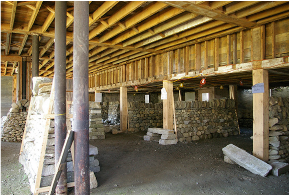
Fig. 3.12 Training walls in the indoor training barn at the Stone Trust Centre, Dummerston, VT, image by Stone Trust staff.
