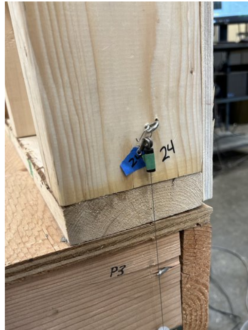
b) Crack slightly more visible/apparent
