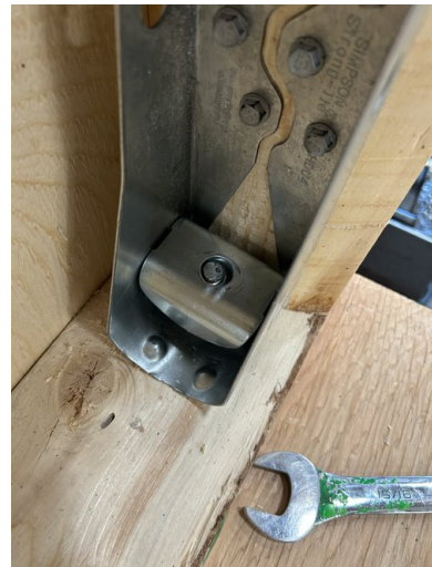
f) Right side hold down (hold down warper, washer to be hammered back into place)
