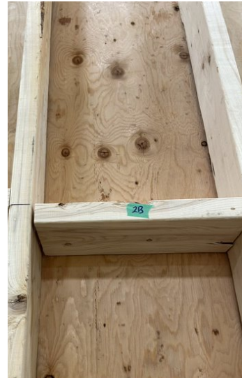
c) General imperfections: gaps in blocking, protruding nails
