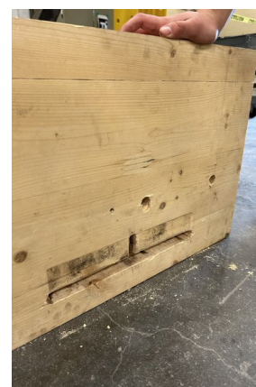
g) Right side connection slot (no visible damage)
