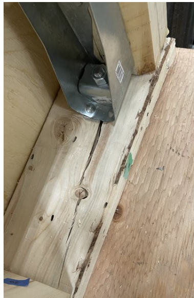
e) Right side hold down (bottom plate splitting due to uplift)
