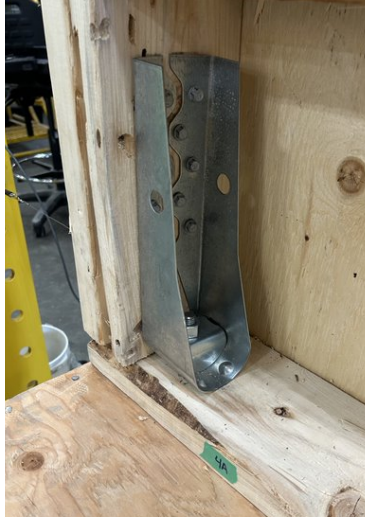
b) Left side hold down (no damage development on inside of hold down)
