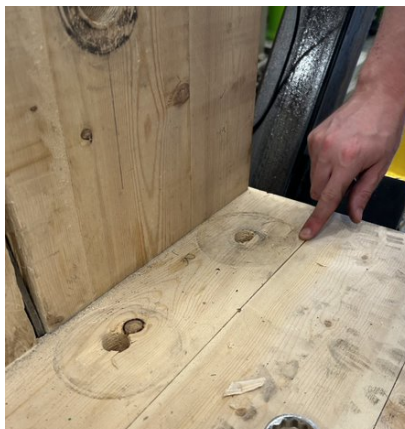
f) Hold down bolts (upgraded washers to mitigated uplift between base and grade beam)
