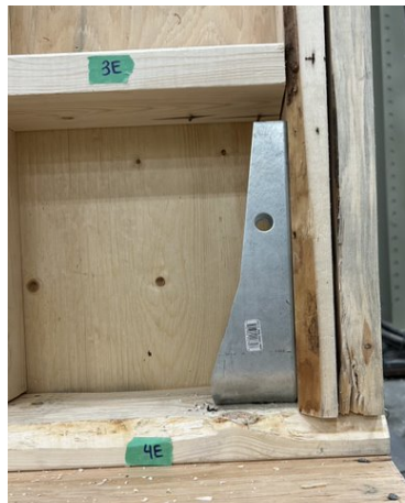
e) Right side hold down (near 4E); note lumber defects
