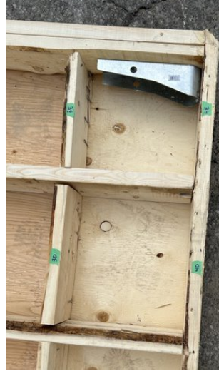
b) Studs pulling out of bottom plate
