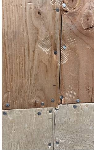
b) Nails along sheathing panel joints pulled in
