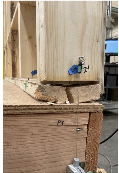
f) Right side hold down (bottom plate cracking at end grain & nail withdrawal between studs and bottom plate)
