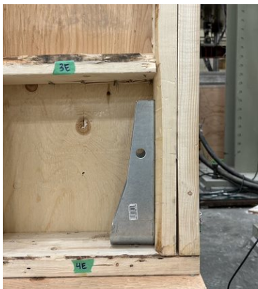
g) Right side hold down (slight gap between double end studs)
