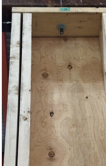
b) Gapping along the double stud due to warped lumber
