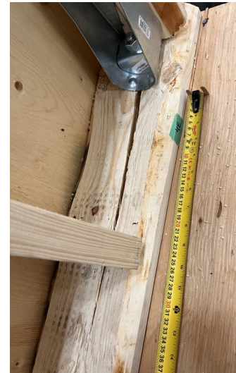
f) Crack in bottom plate
