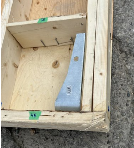
a) Right hold down corner damage
