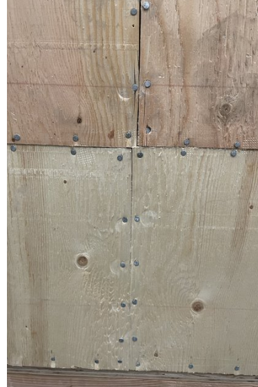
c) Intersection of plywood sheathing (not aligned)
