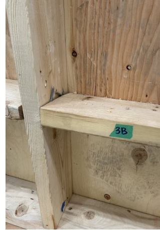
c) Protruding nails
