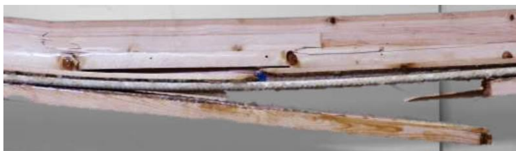
(e) Crack detail (front view)
