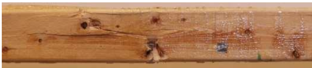
(e) Crack detail (bottom view)
