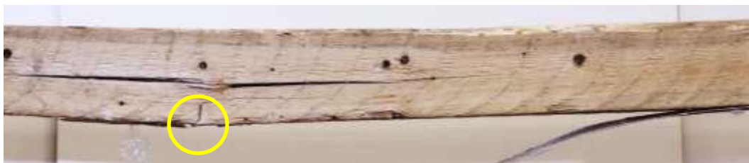
(c) Crack origin detail (back view, mirrored)
