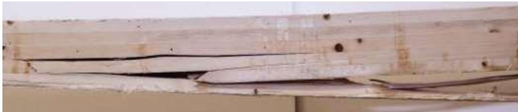
(c) Crack detail (front view)
