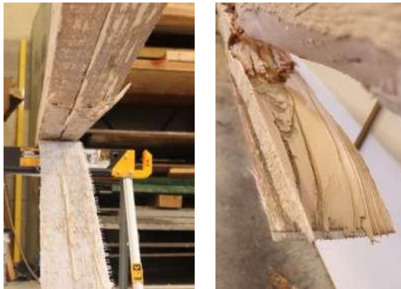
(a) Wood-FRP debonding
