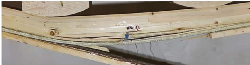
(c) Little-to-no bonded resin at midspan
