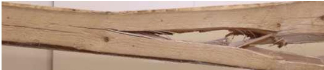
(c) Crack origin detail (back view, mirrored)
