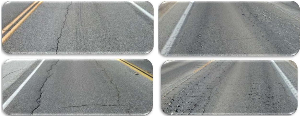
Figure 3. Alligator Cracking A (Left Column) and Alligator Cracking B (Right Column) (Feldman et al., 2015)
