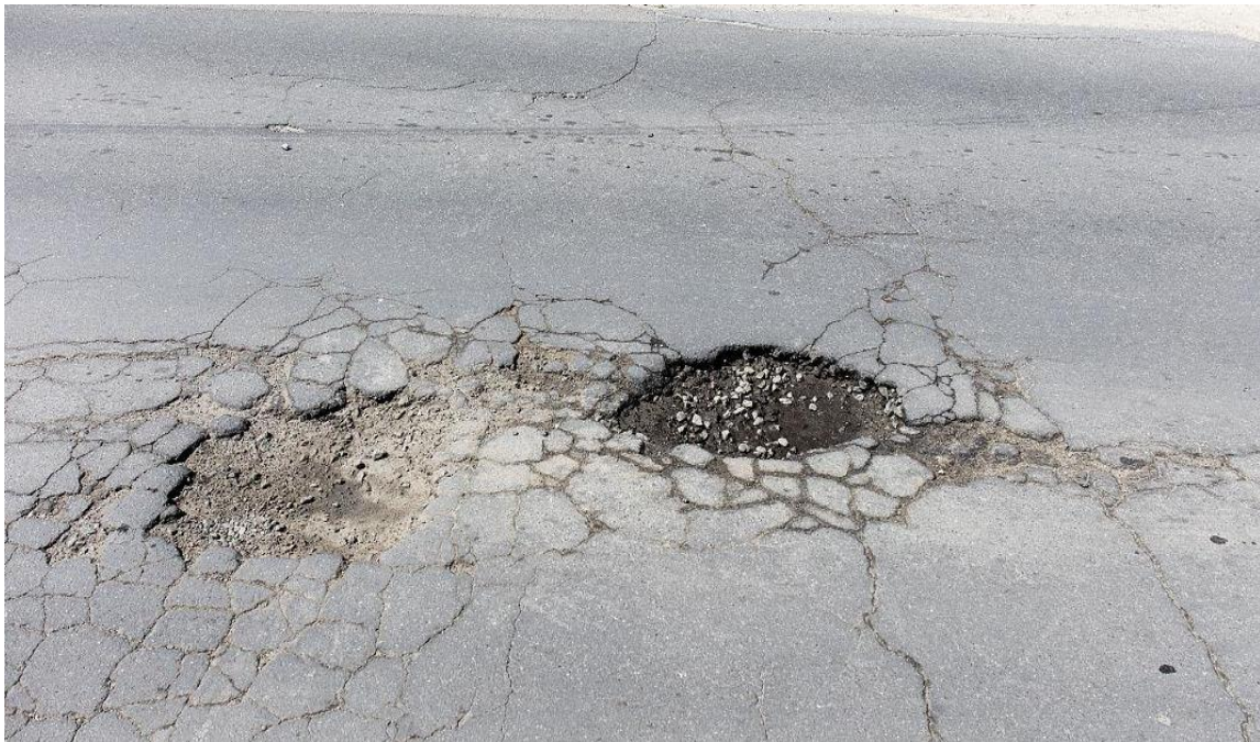
Figure 5. Potholes on Flexible Pavement
