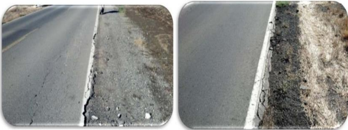
Figure 4. Edge Cracking (Feldman et al., 2015)
