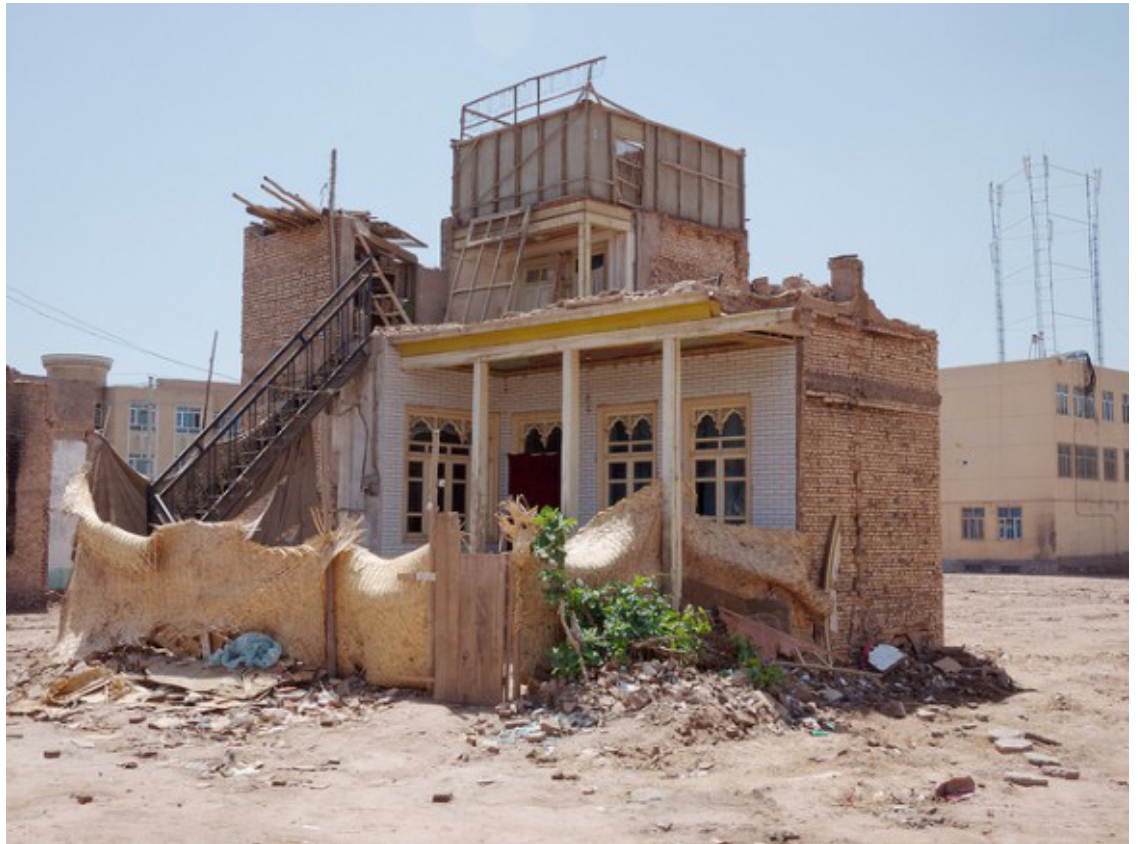
Fig.4-3-5 Old City of Kashgar under demolition in 2014. Photograph by Far West China. 7
