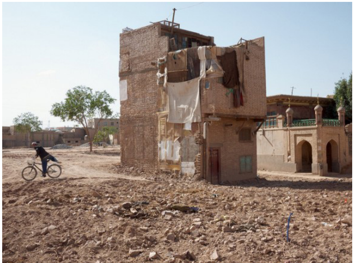
Fig.4-3-6 Old City of Kashgar under demolition in 2014. Photograph by Far West China. 7
