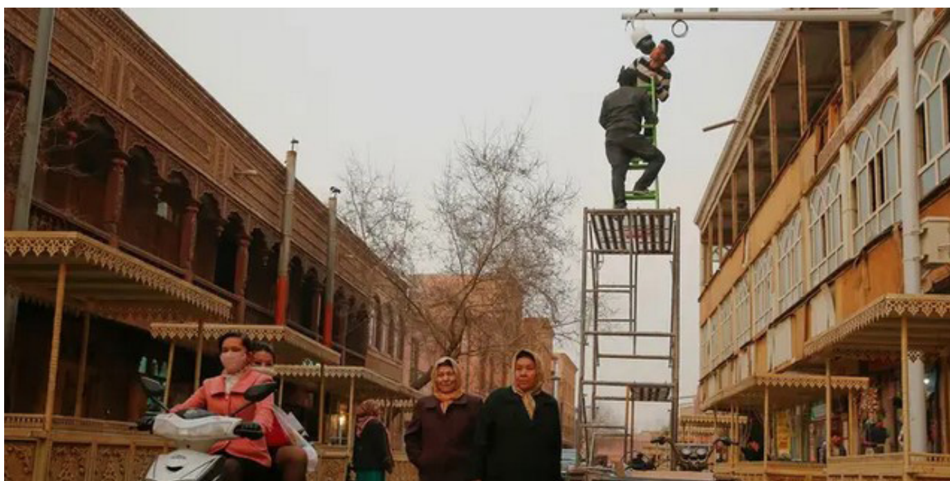
Fig.4-4-26 Men install a CCTV camera in North Jiefang Road Market in the old town of Kashgar, March 23, 2017. 26
