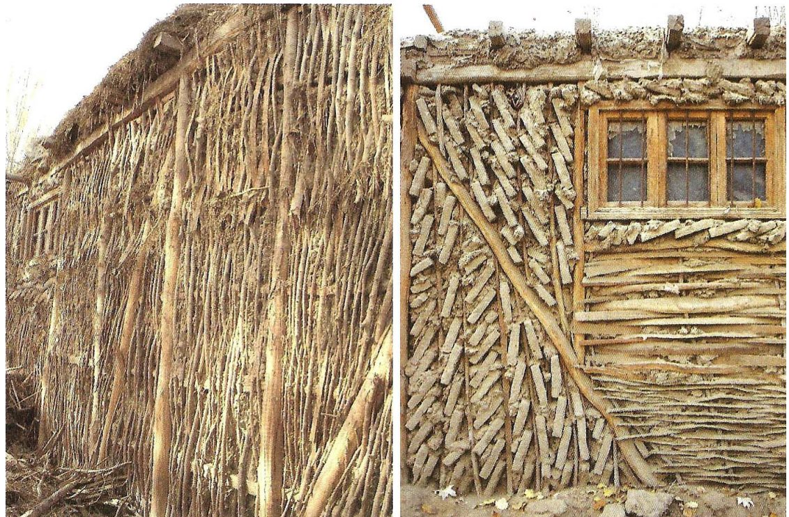
Fig.3-1-5 Appearance of residential walls in Hotan Area. Photographs by Chen Lin. 17
