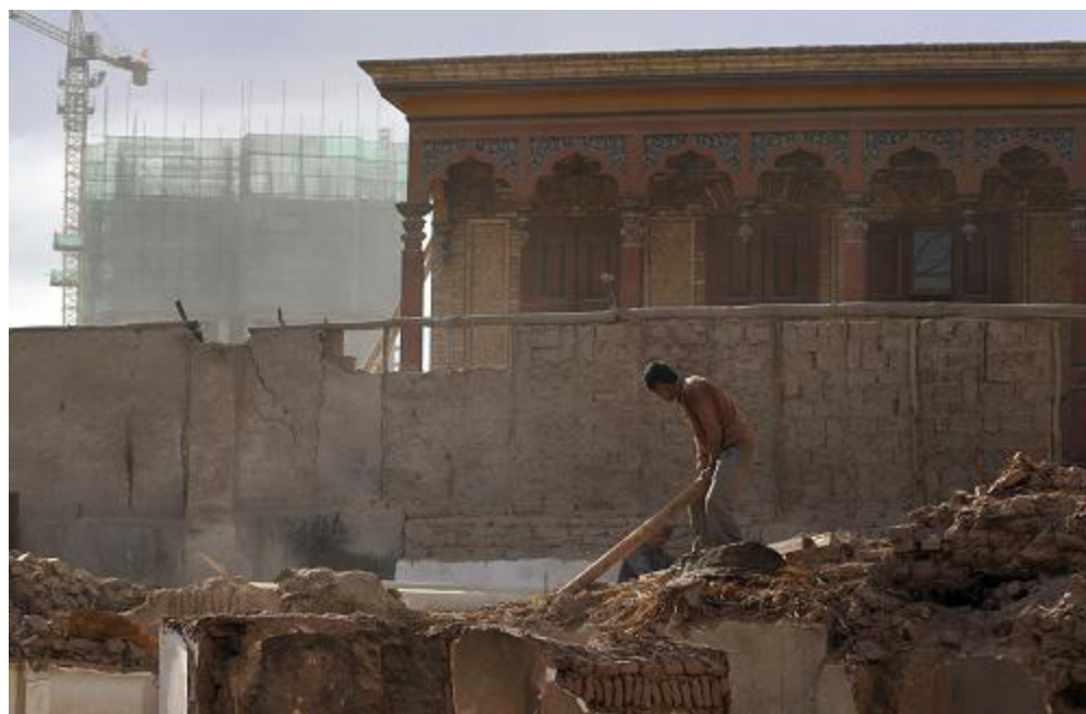
Fig.4-3-13 On June 3, Uyghur residents in the Old City of Kashgar, Xinjiang, were demolishing old houses. Photograph by Shen Qiao, Xinhua News Agency reporter. 12
