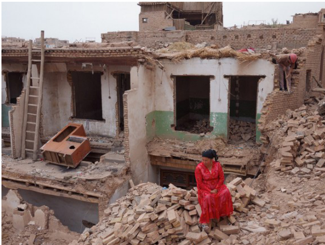
Fig.4-3-7 Old City of Kashgar under demolition in 2014. A woman sits on the rubbles. Photograph by Far West China. 7
