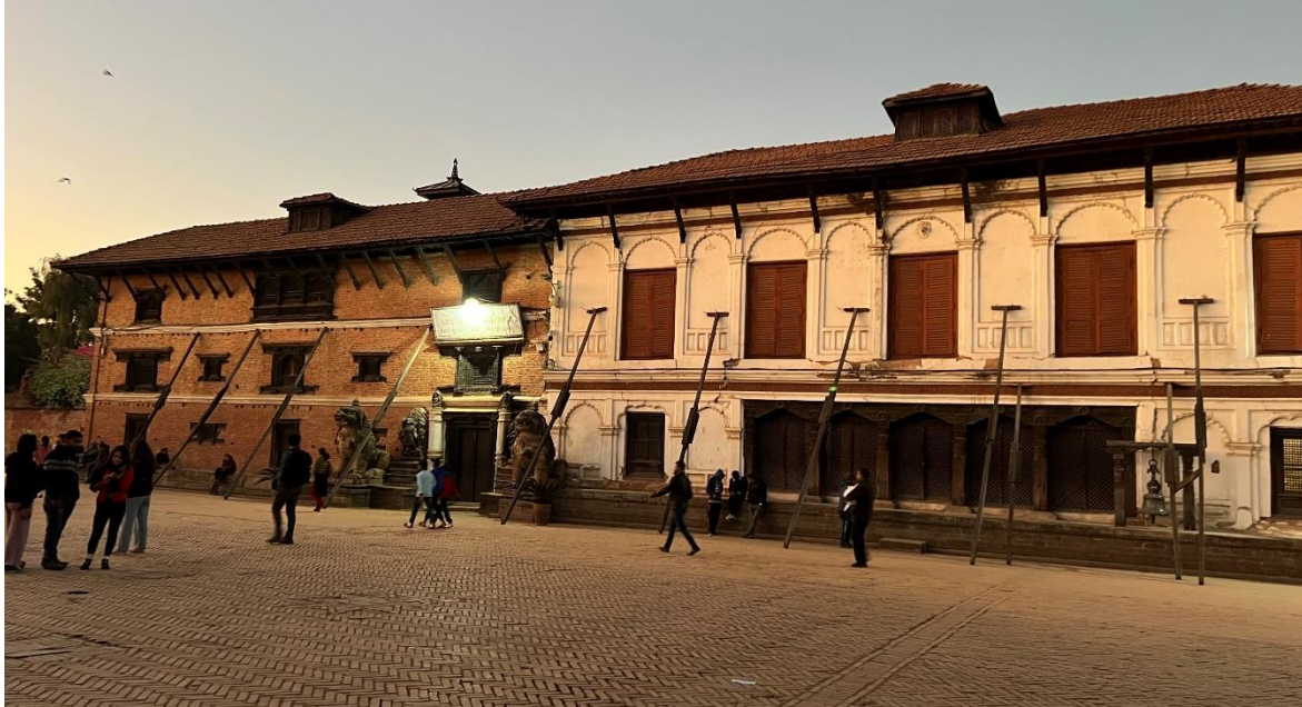
Figure 12. Heritage Building Still Under Construction in December 2022 in Bhaktapur Durbar Square. (Field Data, 2022).
