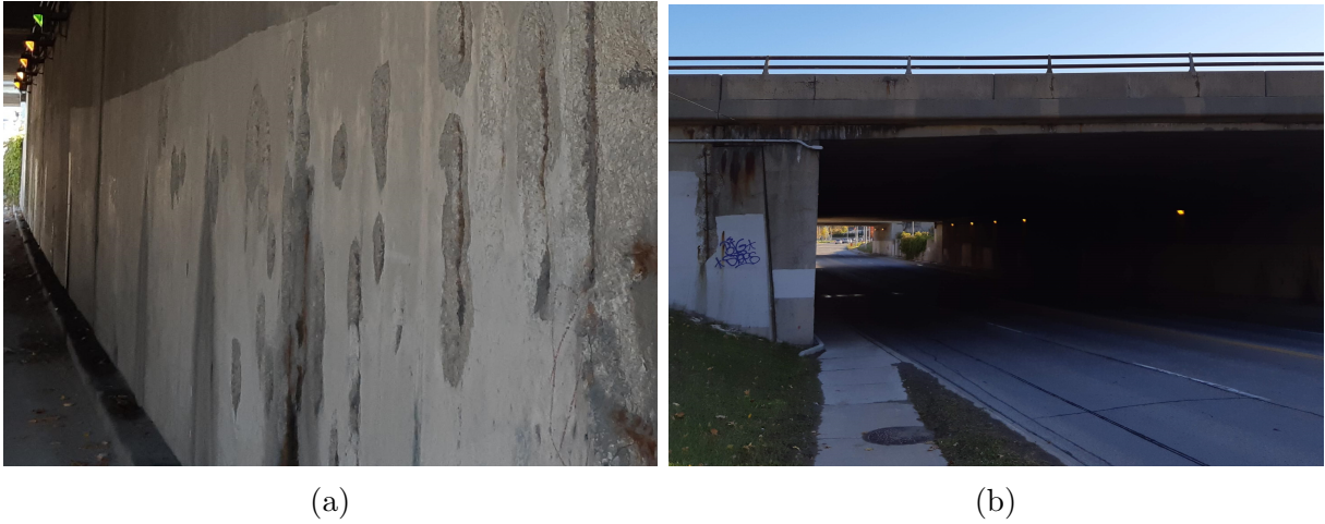
Figure 3.9: Overview of test spalling regions at a bridge abutment (a) underneath bridge (SA) and (b) outside bridge (SB).
