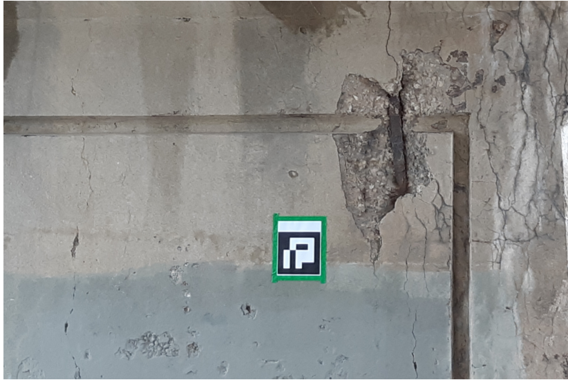
Figure 5.12: Fiducial marker taped to bridge’s surface near spalling region 1 to quantify spatial alignment error in MSL for panoramic image localization.
