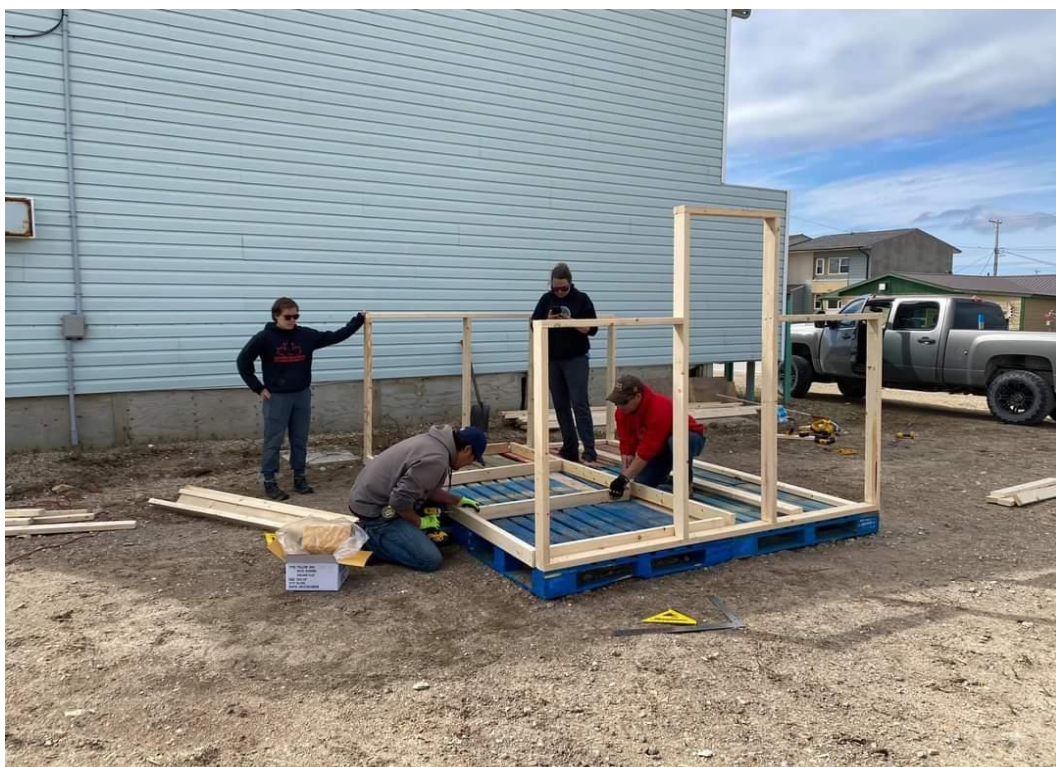
Figure 18: Construction of a greenhouse donated by the operators of the local hydroponic unit. Source: Mitchell, 2021
