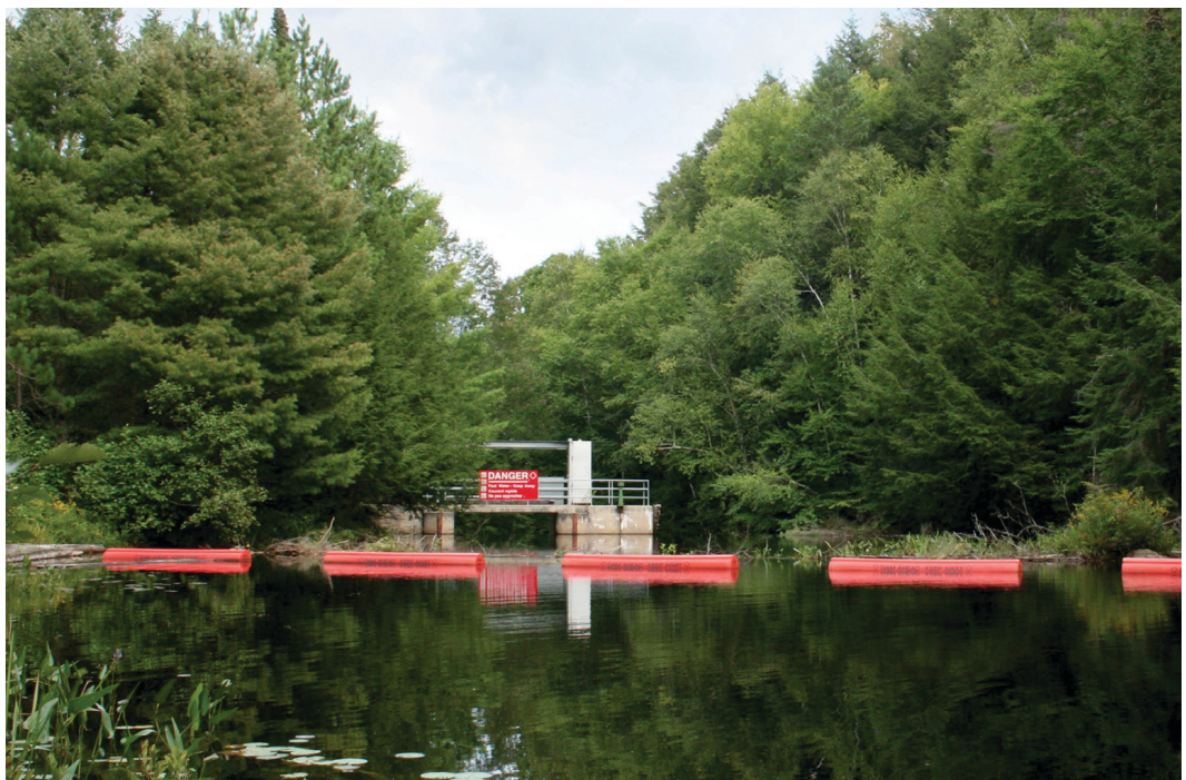
Fig. 1.13 Upstream view of the Cache Lake dam, August 2023. Non-powered dams like this control tributaries of the Kichissippi that flow through the park.
