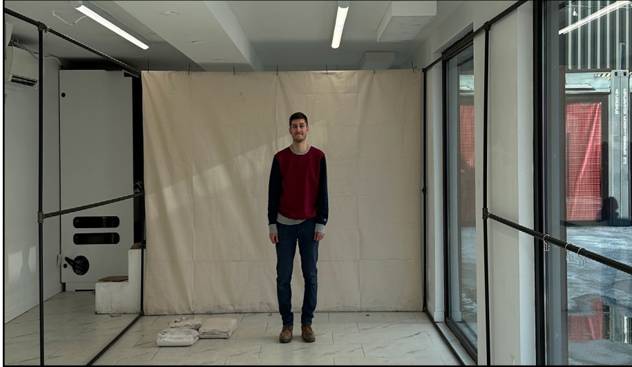
Figure 4.15 Initial Construction Stage of Building the Exterior Shell with Pipes and Attaching Back Fabric Wall. Photo by Author (2024).
