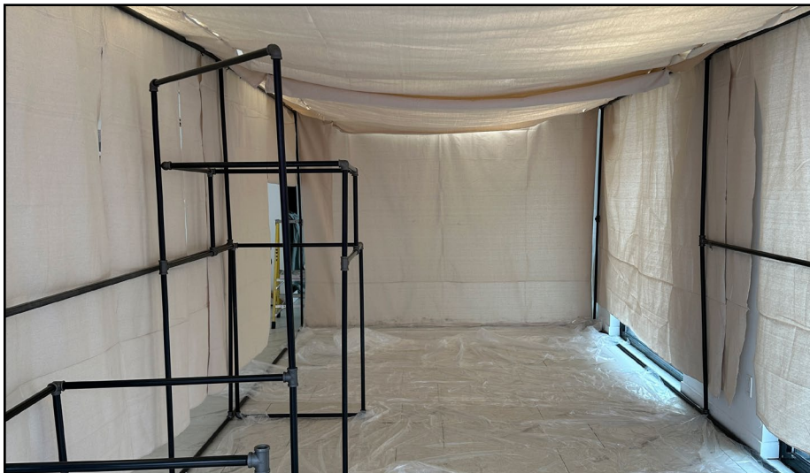
Figure 4.16 Construction Stage with Drop Sheet Installed to Cover entire Structure. Photo by Author (2024).
