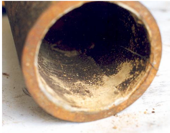
Figure 3-4: Cement mortar lined pipes from the City of Toronto. The pipes were lined in 1969 (top) and 1979. The pictures were taken in 1998. They show excellent long-term performance of the cement mortar lining (pictures courtesy of Kamran Sarami).
