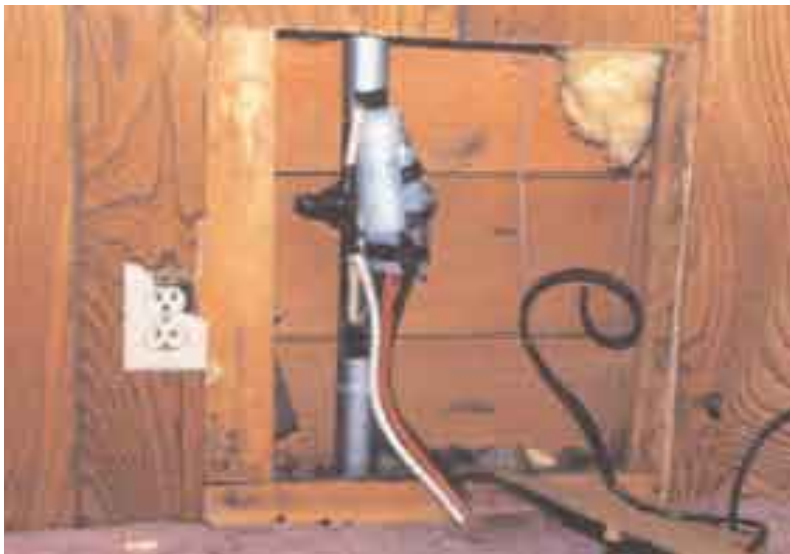
Fig. 5.84: Photo of electrical tampering in a typical grow house
