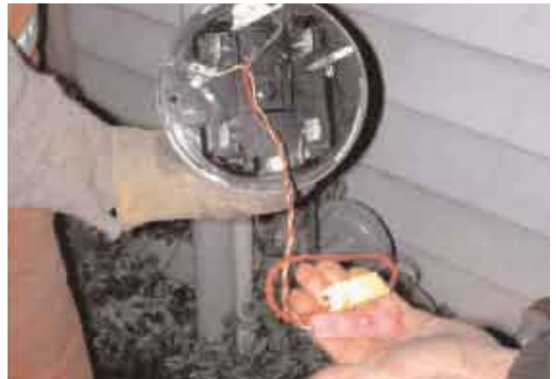
Fig. 5.85: Photo of electrical tampering in a typical grow house
