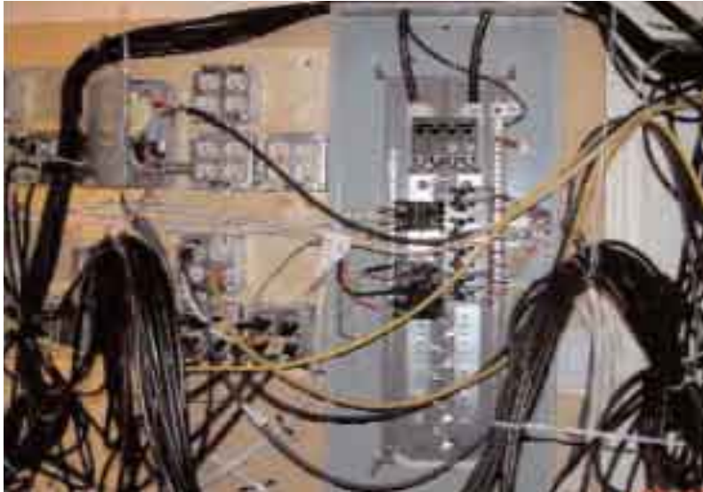
Fig. 5.82: Photo of electrical tampering in a typical grow house
