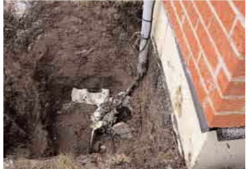
Fig. 5.83: Photo of electrical tampering in a typical grow house
