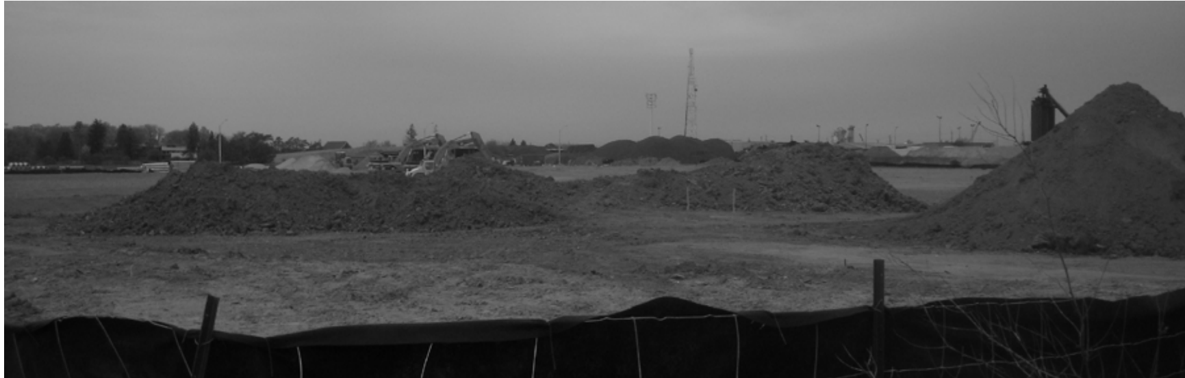
Fig. 1.11: Construction site at the corner of Midland Avenue and McNicol Road, December 2004
