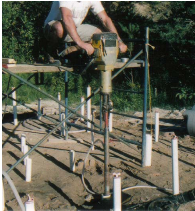
Figure 2.5. Photograph of use of jackhammer to push steel casing for installation of CO 2 injection wells.
