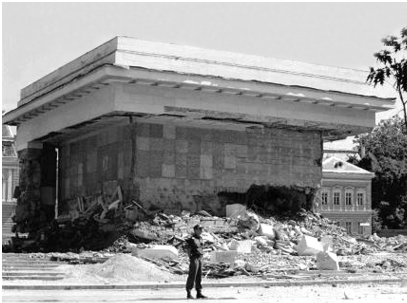
Fig.2.29. After years of wrangling over what to do with the mausoleum, the government decided to knock it down. After three attempts to demolish it with explosives, the 1.5m thick walls of the structure still stood. .
