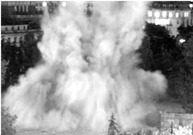
Fig.2.30. In desperation, the structure was demolished using smaller detonations and mechanical gear, finally collapsing the mausoleum to the ground.
