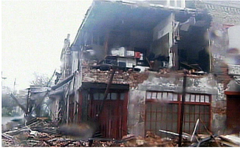
Figure 1.7 Damaged building due to Hurricane Katrina, New Orleans (CNN, 2005)
