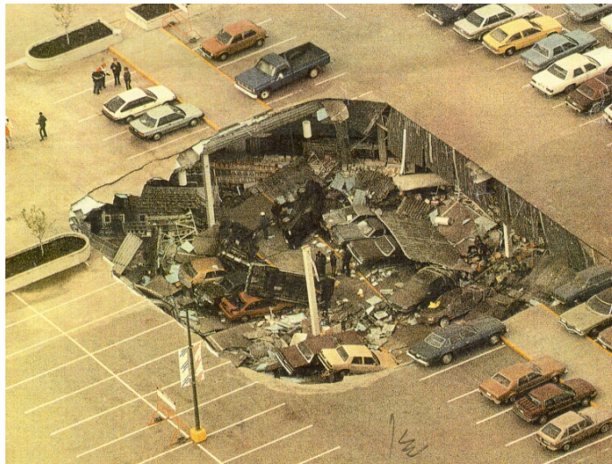
Figure 1.1 Save-on-Foods Grocery Store failure, Canada (Closkey, 1988)
