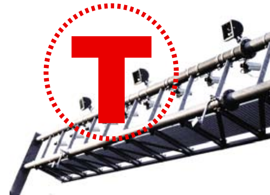
Figure 63 - Gardiner Expressway Toll System gantry
