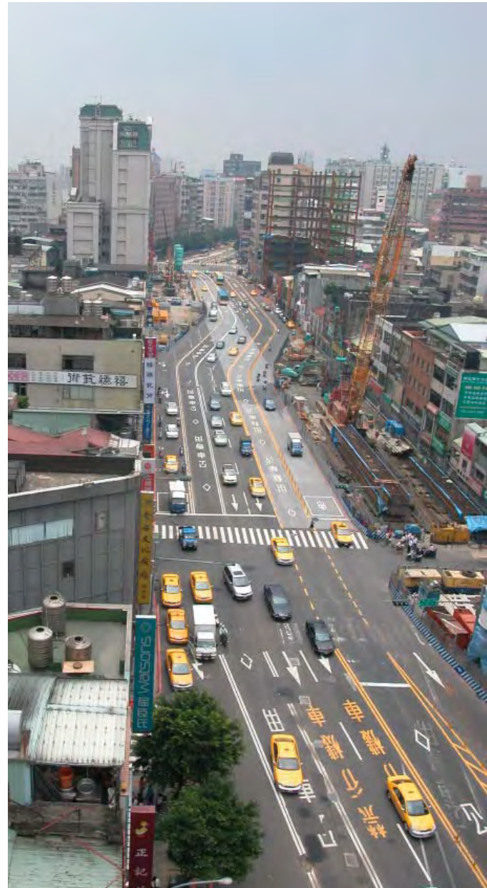
5.11 looking West on Shinyi Road, with the construction of the new subway line [05.2005]
