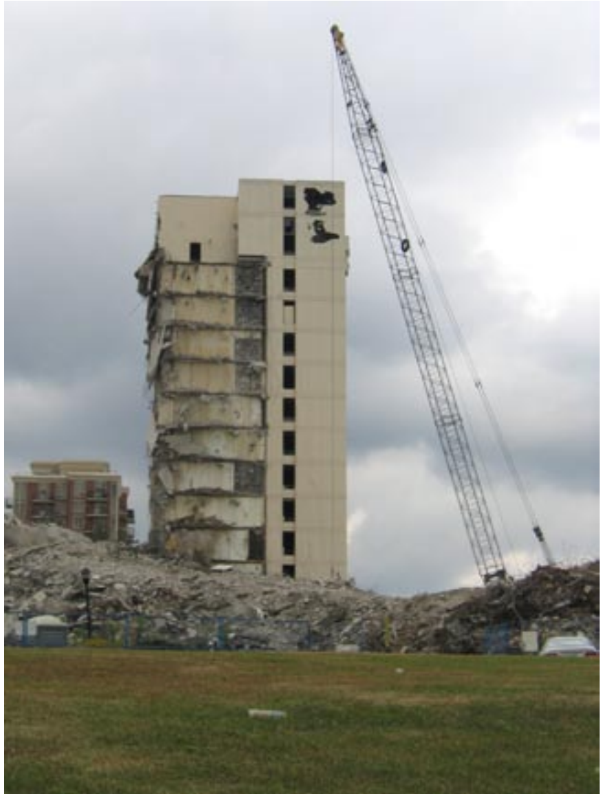
0.1 Demolition in Progress August 2006 Former 'Inn on the Park', Leslie St. & Eglinton Ave., Toronto
