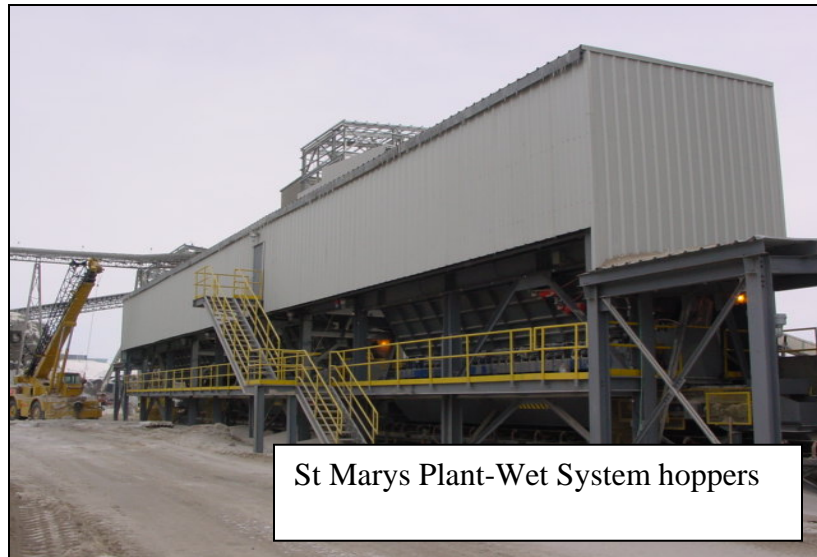
Figure 15: Wet System Hoppers at St Marys Plant Grate Cooler
