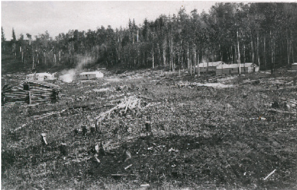
149(Below) Construction Photograph - View of Worker's Camp Showing the Extent of Trees Cleared
