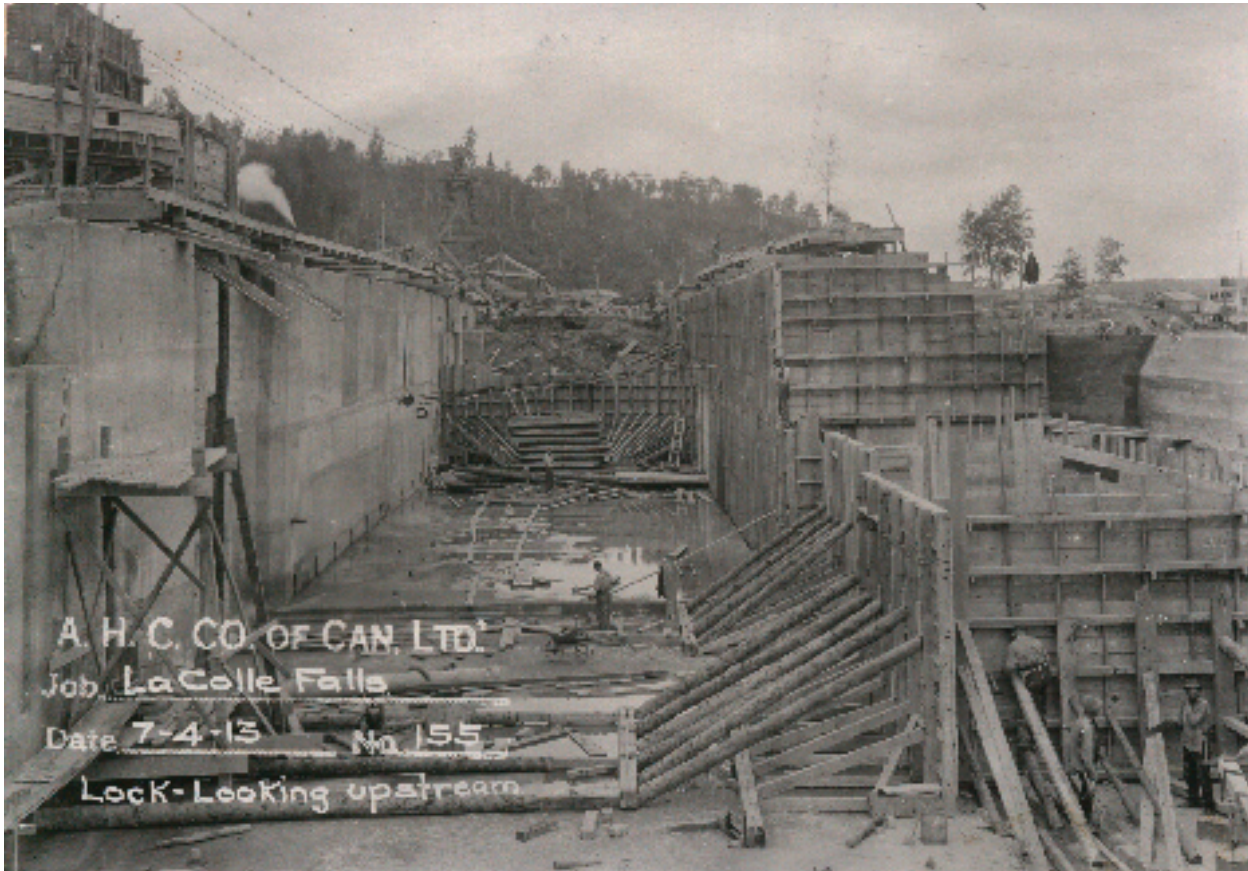
119(Above) Construction Photograph #155 - View of Shipping Lock Looking Upstream Showing Completed South Wall Formwork for North Wall
