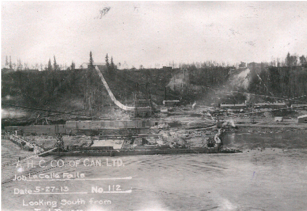
89 Construction Photograph - Panorama - # 112 and #113 - This View Shows the Entire Construction Site, the Coffor Dam is Visible in the River, Behind it is One Full Wall of the Shipping Lock. At the Top of the Hill is the Construction Camp. Concrete was Mixed in the Building at the Top of the Hill, and Poured Down the Wooden Chute to the Site Below.
