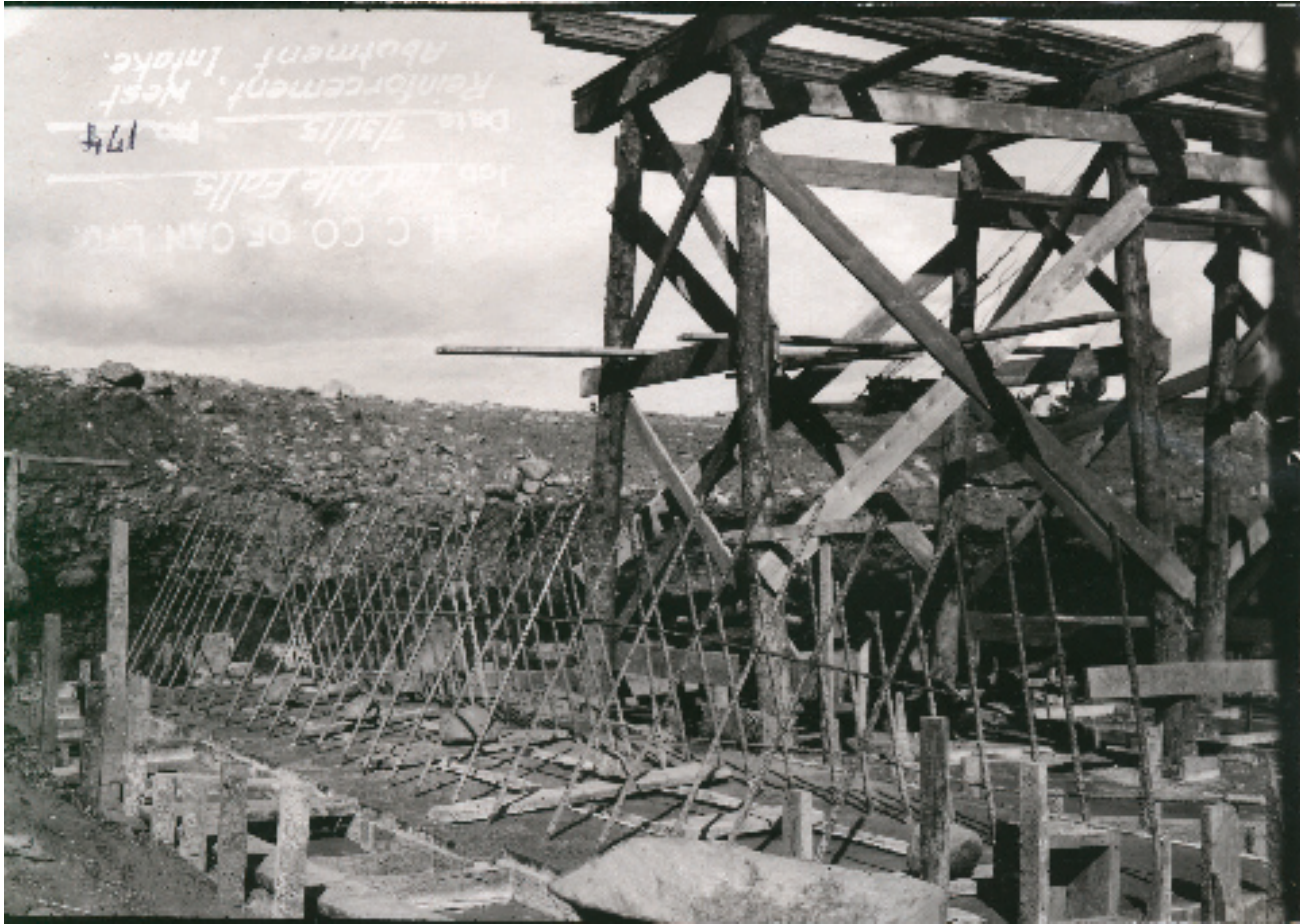
134 Construction Photograph - Panorama - #174 - Reinforcement, West Abutment Intake, and #175 - Concrete on Intake Floor
