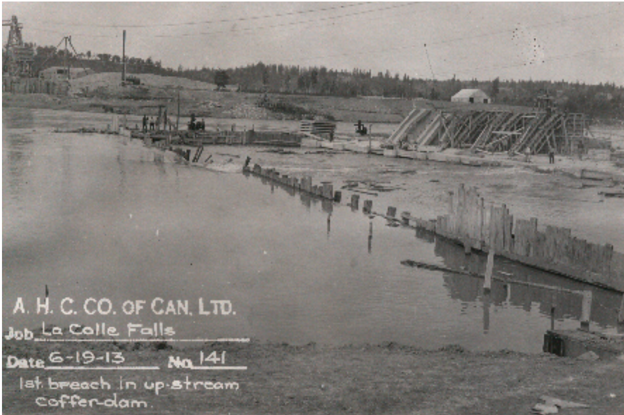
109(Below) Construction Photograph #141 - First Breach in Up-Stream Cofferdam - the First Step in Removing the Wooden Cofferd Dam was to Remove Boards and Allow the River Water to Enter
