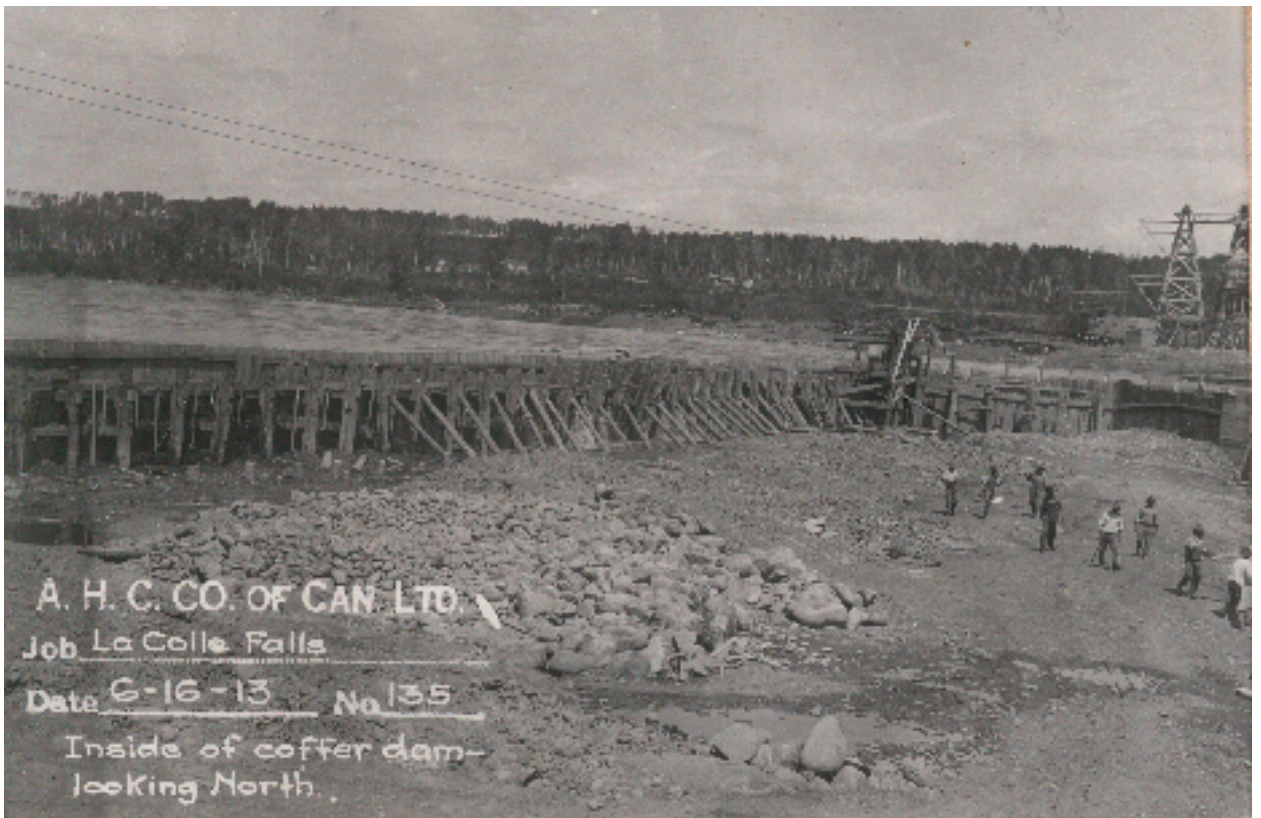
105 Construction Photograph #135 - View of Inside of Wooden Cofferdam Holding Back the River Water Showing Exposed Riverbed
