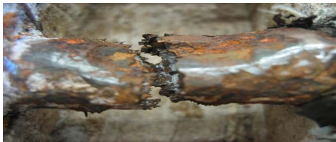
Figure 3.15 Flexural fatigue failure by steel rupture
