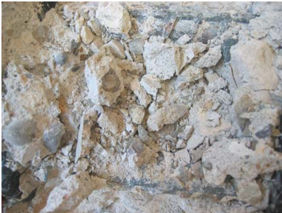
a) Concrete above the steel bar
