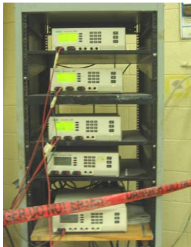
a) Power supplies
