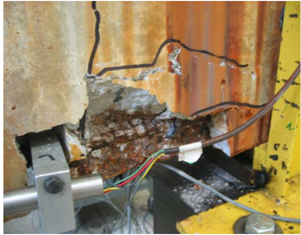
b) Concrete cover spalled for corroded beams
