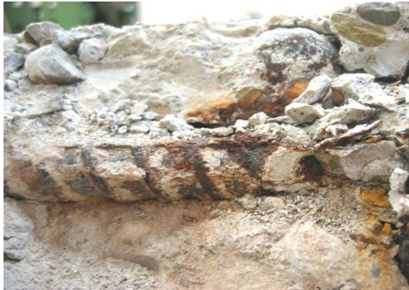
Figure 3.20 Traces of the condensed concrete in front of the steel bar lugs
