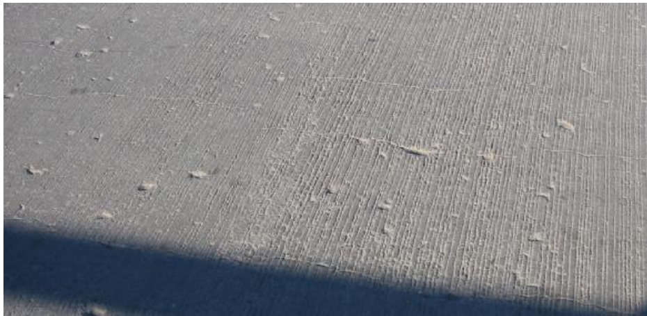
Figure 4. 94. Pop-outs on the surface of the bridge deck.
