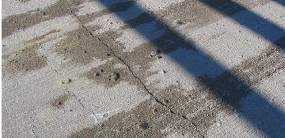
Figure 4. 93. Longitudinal cracks on bridge deck.
