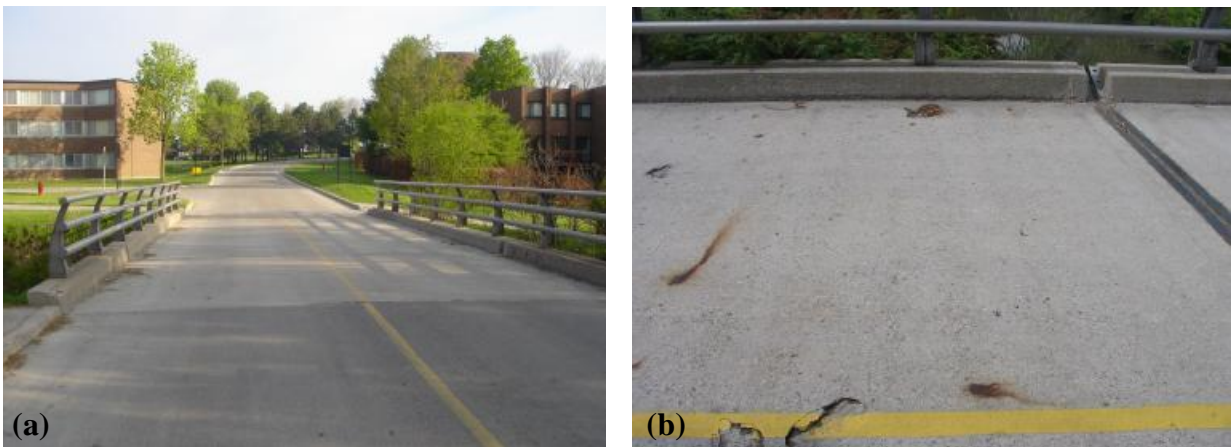
Figure 3. 22. (a) A view of the bridge at the University of Waterloo, (b) some of the deteriorated spots on one of the approaches.
