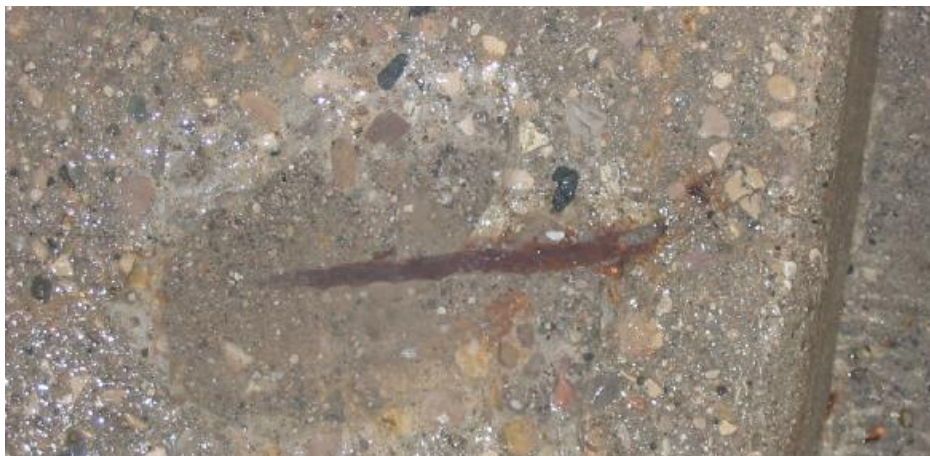
Figure 4. 95. Corroded steel rebar in the one of the sidewalks.
