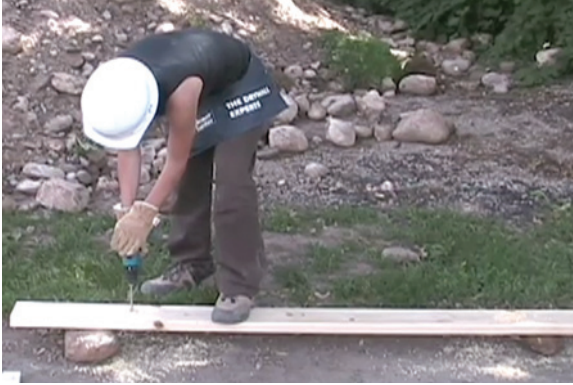
Left: 2.168 Drilling a hole in a sill plate at an anchor bolt location.
