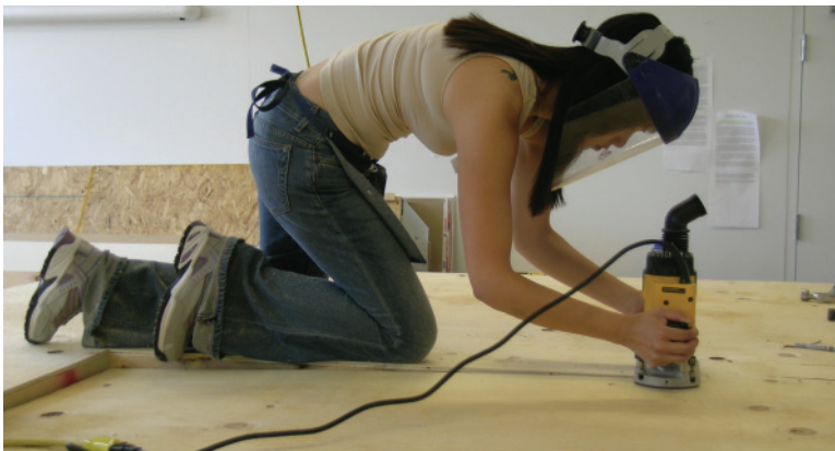
Left: 2.112 Using a router to cut out the sheathing at a window opening.
