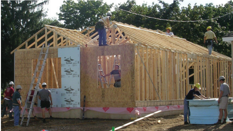
Left: 2.249 The third house with the walls and roof trusses erected by a group of Mennonites in one day.
