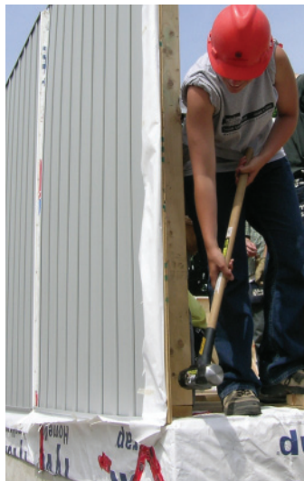
Far Left: 2.200 Ensuring that two wall panels are aligned properly on the exterior of the house.
