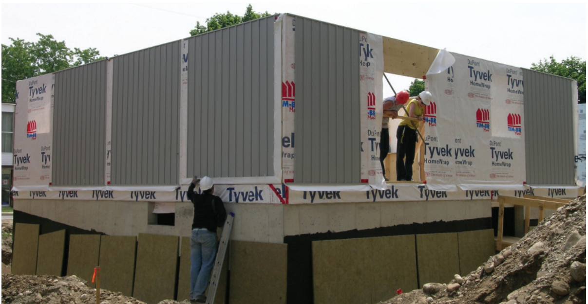
Below: 2.202 View of the completed walls from the exterior of the house.
