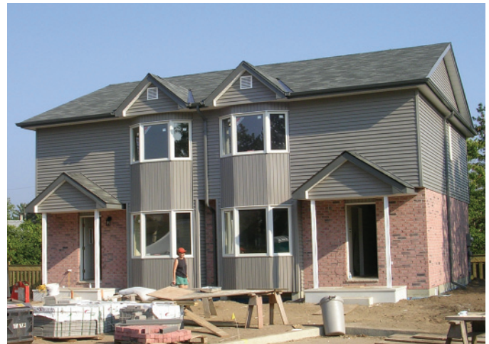
Top Left: 1.32 Ted trims a prefabricated wall panel for the bay window.
