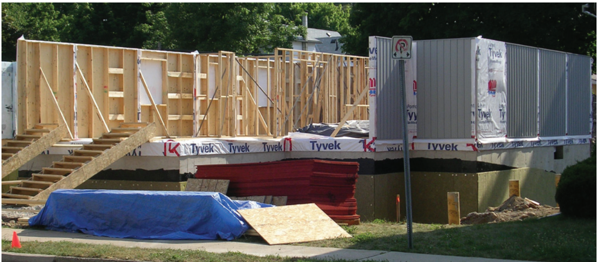
Below: 2.210 View of the erected walls at the end of the day.
