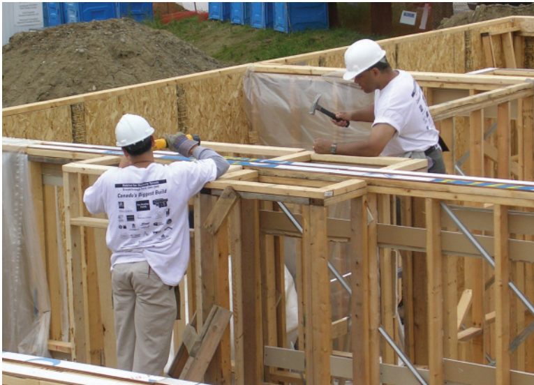
Above Left: 1.18 Additional framing inserted to fill the gap between a SIP and the gypsum board break at a party wall.
