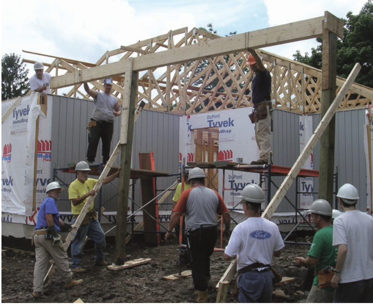
Left: 2.232 The posts are over nine inches too high when they, and the beam at the front of the carport, are erected.
