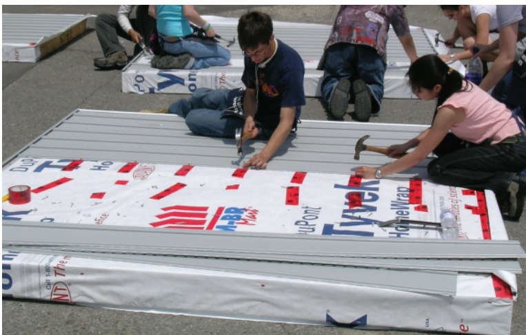
2.142 Removing incorrectly installed siding panels.
