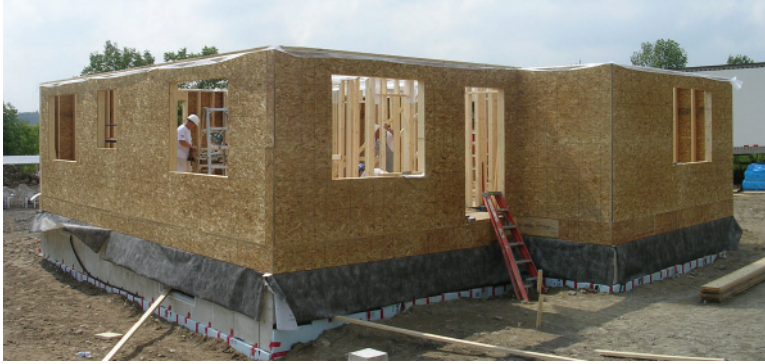
1.23 All walls are erected and capped by the end of day four.
