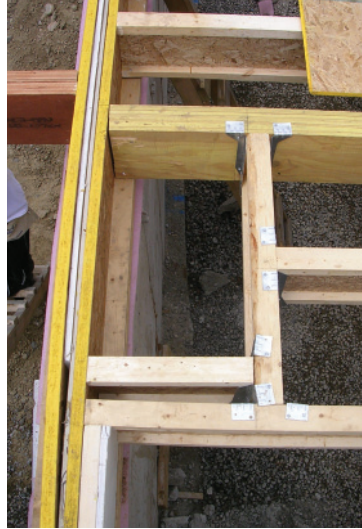
Far Left: 1.13 A mechanical chase cut out of the floor sheathing. Left: 1.14 A mechanical chase that was corrected before the installation of the floor sheathing.
