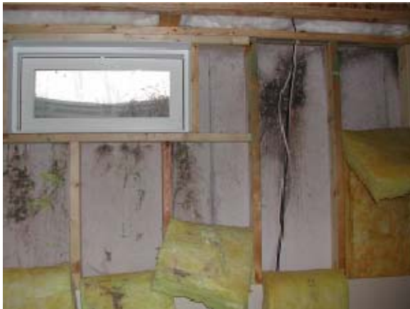
Figure 3.22: Mold growth on upper portion of basement wall
