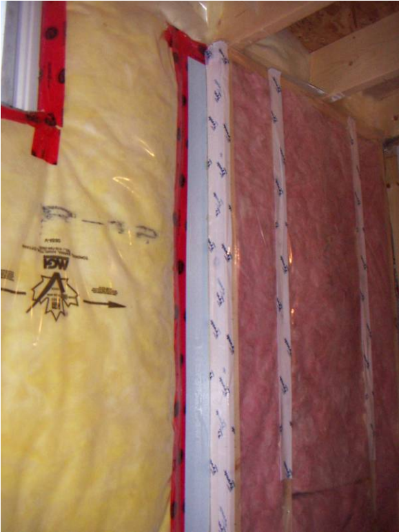
Figure 7.15: Taping of perimeter studs, and faces of inner studs (at staple holes)
