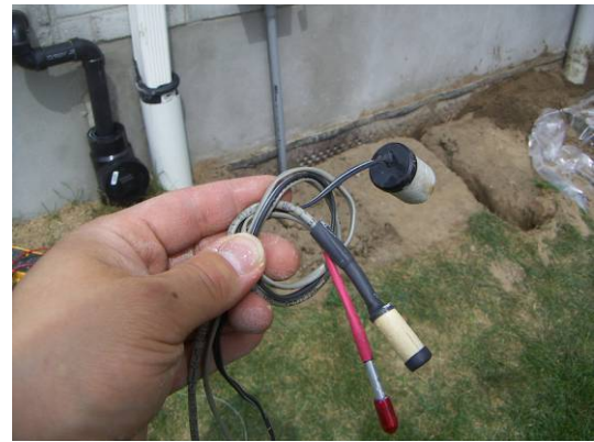
Figure 5.49: Gypsum soil block, wood plug sensor, and temperature sensor in soil installation
