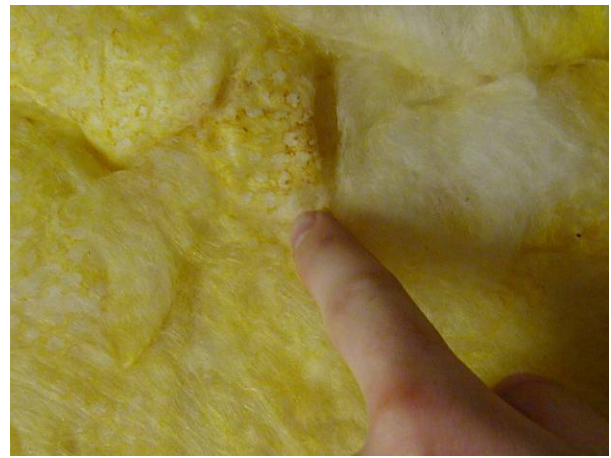
Figure 6.76: Small brown stains in June 2004; double polyethylene wall (panel 2)
