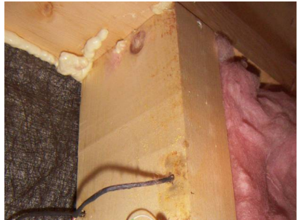
Figure 7.27: Brown staining at inboard side of upper portion of right-hand test bay stud
