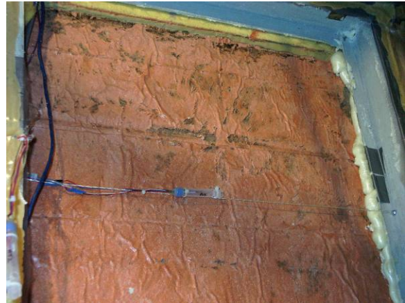
Figure 4.15: Deterioration of wall-side waterproofing coating (Goldberg and Gatland 2006)
