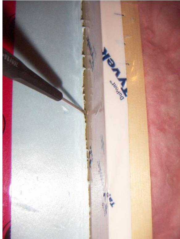
Figure 7.16: Tape only covers exposed portion of edge studs; could not apply at buffer panels
