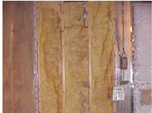
Figure 6.78: Brown stains on interior of fiberglass (panel 2), July 2006
