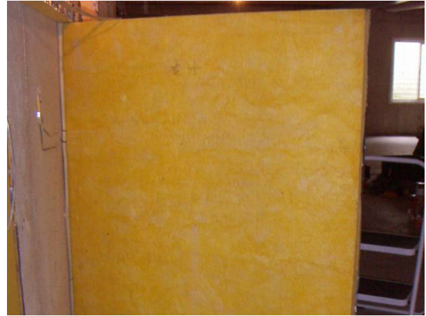
Figure 6.80: Concrete interface of rigid fiberglass in PA-6 wall (panel 7)
