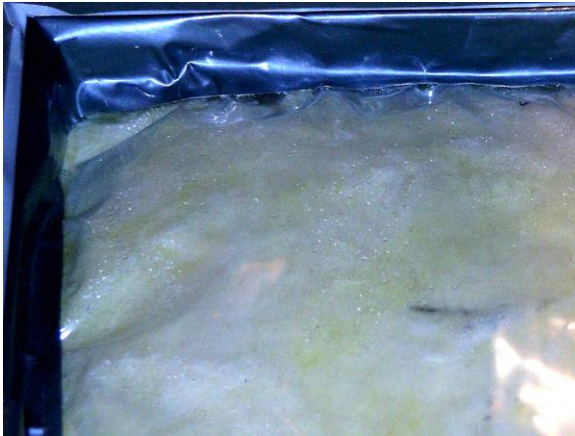
Figure 4.14: Example of worst condensation seen on PA-6 vapor retarder (Goldberg and Gatland 2006)
