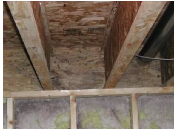
Figure 3.23: Mold growth at insulated rim joist of basement
