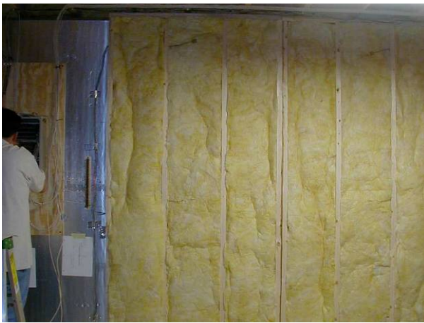
Figure 6.75: Initial condition of interior of fiberglass (panels 1 and 2), September 2003
