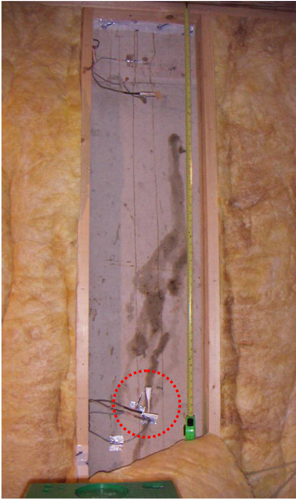
Figure 6.62: Upper portion of wetting plume in single polyethylene wall (panel 1)
