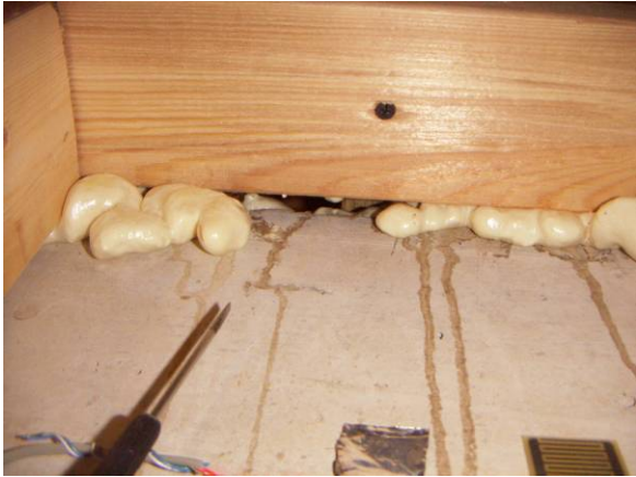
Figure 6.27: Gap in air seal at the top of panel 1
