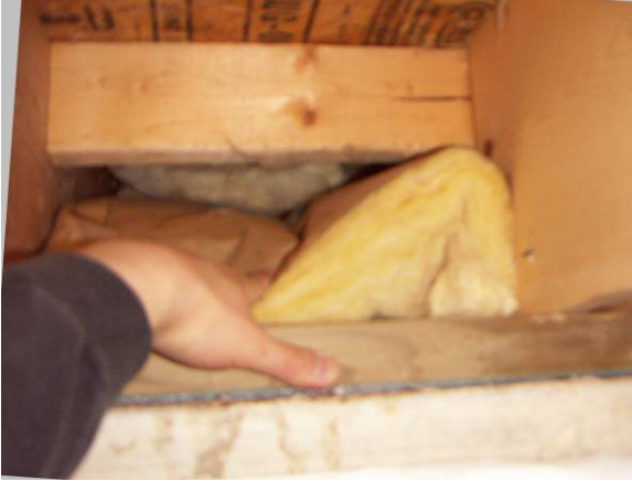
Figure 6.17: Bay interior near Wall 8, showing incomplete blocking/air leakage location
