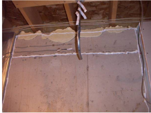
Figure 6.31: Caulk air seal around the perimeter and at form board extension intersection
