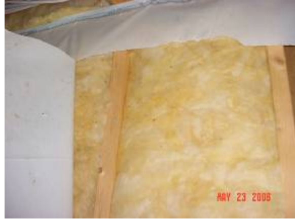
Figure 3.26: Surface mold at interface of fiberglass batt and polyethylene
