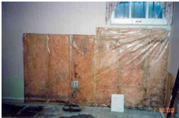
Figure 3.24: Moisture accumulation and mold growth in single polyethylene wall
