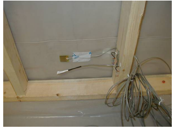
Figure 5.23: Instrumentation package at lower location of stud frame walls (Wall 2)
