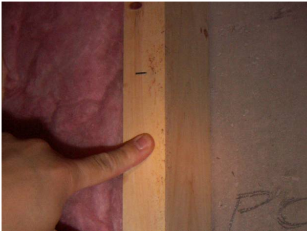
Figure 7.26: Brown staining at inboard side of upper portion of left-hand test bay stud
