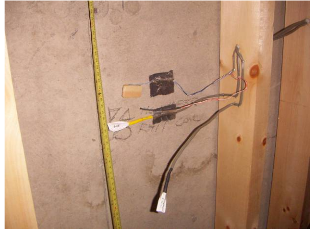
Figure 29: Mid-height sensors in Kitchener basement
