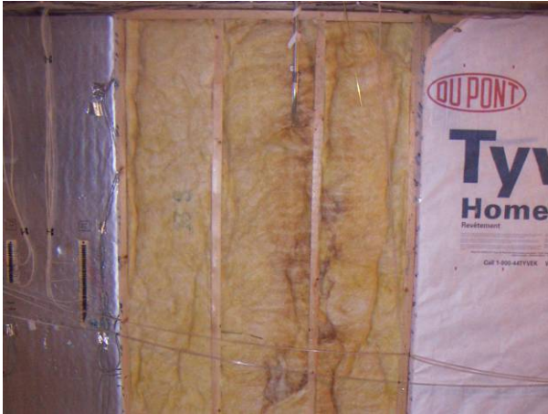
Figure 6.79: Brown stains in XPS/FG (panel 5), July 2006
