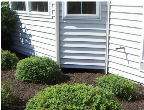
Figure 6.15: Bay near Wall 8, showing shading on above-grade portion of concrete
