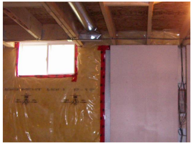
Figure 7.12: Interior view of basement window, for vertical reference, compared to test panels
