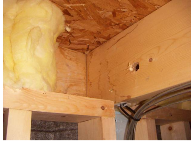
Figure 5.52: Evidence of rim joist moisture damage at Kitchener site
