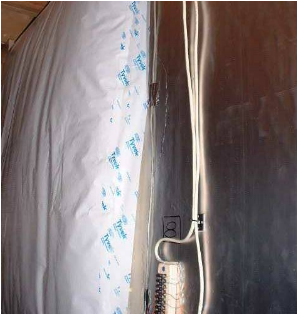
Figure 6.39: Roll blanket lateral seal failure in October 2003
