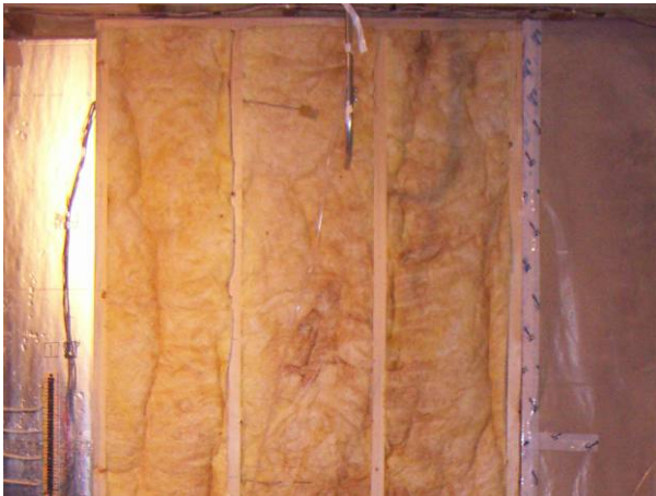
Figure 6.77: Brown stains on interior of fiberglass (panel 1), July 2006
