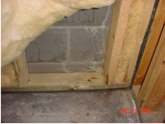
Figure 3.25: Moisture accumulation behind polyethylene; high MCs in framing
