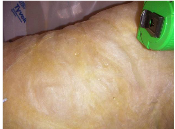
Figure 6.65: Water beading at fiberglass batt in double polyethylene wall (panel 2)
