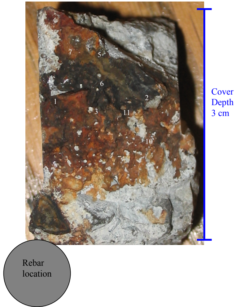
Figure 73: A photograph showing the distribution of corrosion products at a crack in the dynamically loaded OPCC beam. The Raman spectra from the locations indicated by numbers in this photograph are presented in Figure 74.
