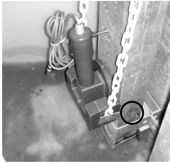
Figure 54: Encircled area shows corrosion products coming out of the casting defect in the submerged region of the dynamically loaded HPC beam 3.
