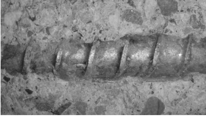
Figure 4-30. Photograph of corroded bar exposed to OPC concrete
