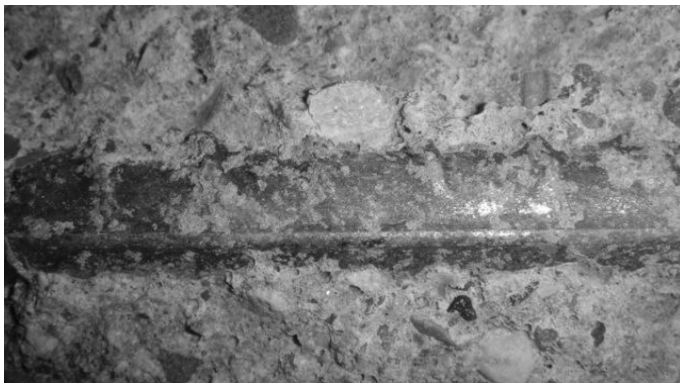
Figure 4-32. Photograph of corroded bar exposed to slag concrete
