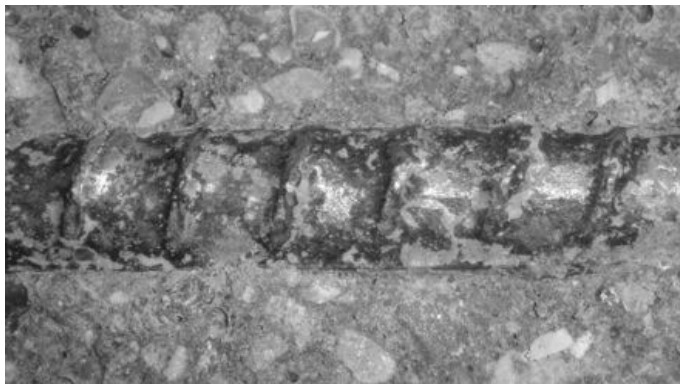
Figure 4-31. Photograph of corroded bar exposed silica fume concrete
