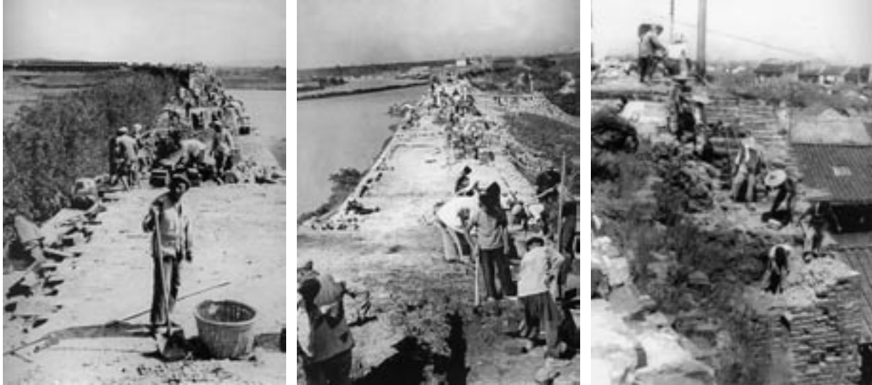
2.15 (Left) De-construction of the Nanjing city wall in the 40s at the Guanghuamen area, (Middle) at the Shuiximen area, and (Right) at the Tongjimen area.
