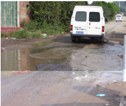
Sewage Leaking on Lingyuan Road
