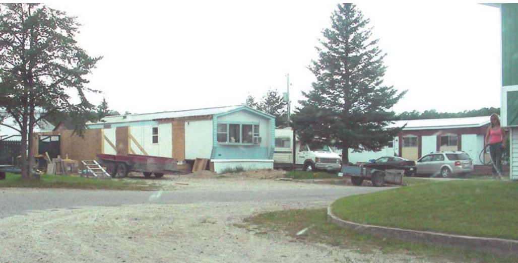
Fig. 2.2 An addition to a small house, during construction. Illustrates desire of residents to improve living environment.
