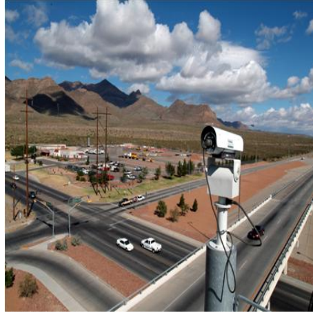
Figure 6.1: Example of a camera mounted on a pole above highways and recording video sequences (Source: Texas Transportation Institute).
