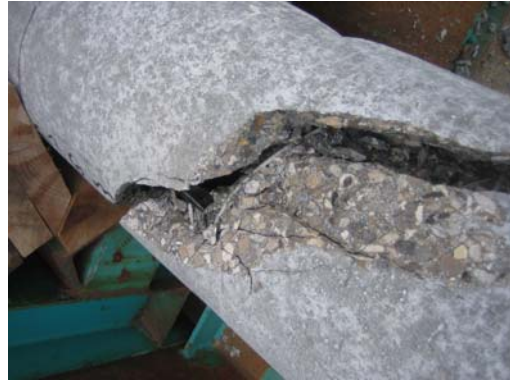
b) Torsional failure showing helical steel
