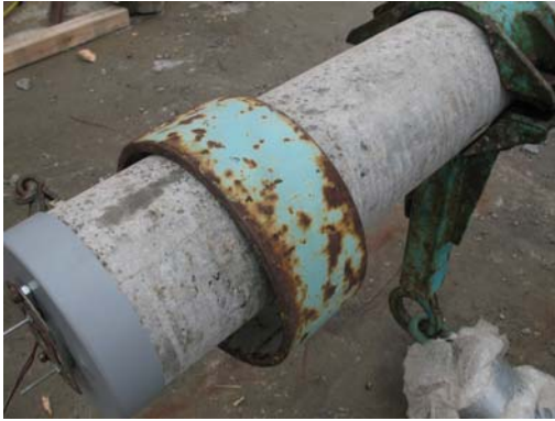
a) Longitudinal transfer crack along strand
