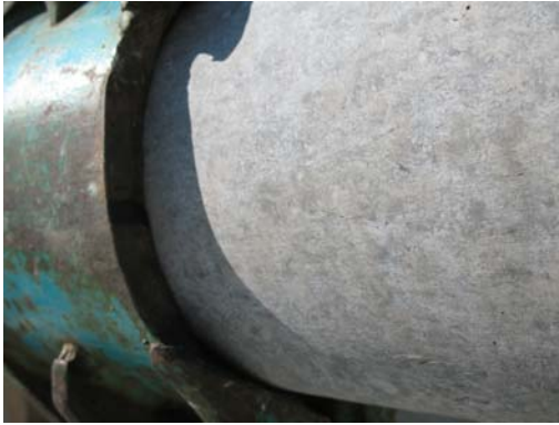
a) Crack due to tightening of collar
