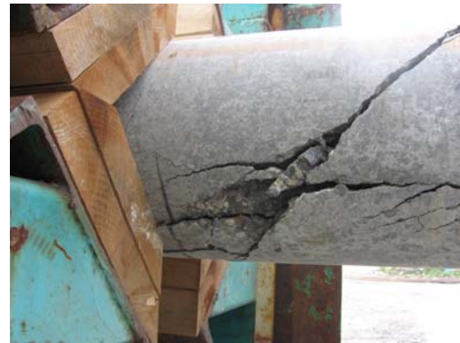
d) Failure at butt (back side)
