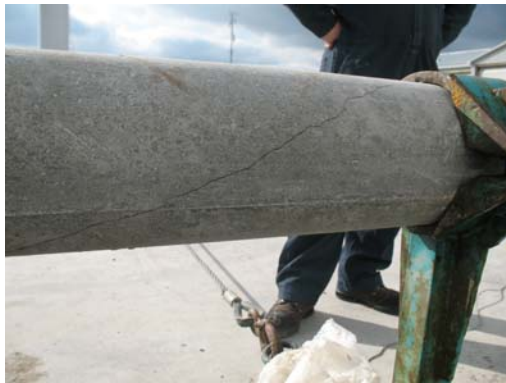
c) Cracking at collar (back side)
