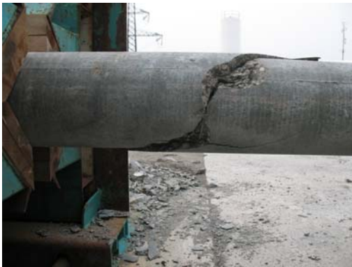
c) Failed section (back side)
