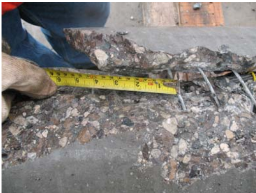
e) Larger spaced helical steel at collar failure location
