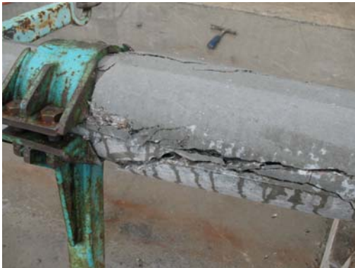
e) Failure and cracking at collar
