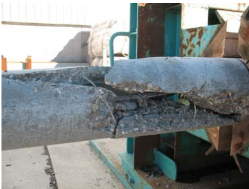
e) Failure (loading side)
