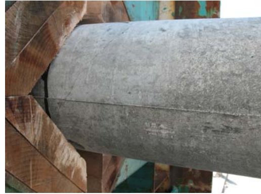
b) Initial cracking at butt
