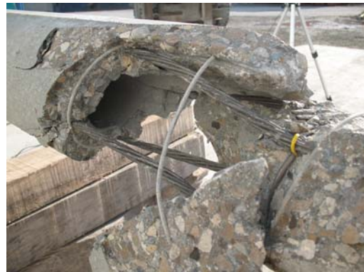
d) Cracking along helical steel
