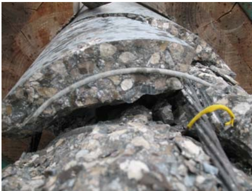
e) Helical steel at failed section
