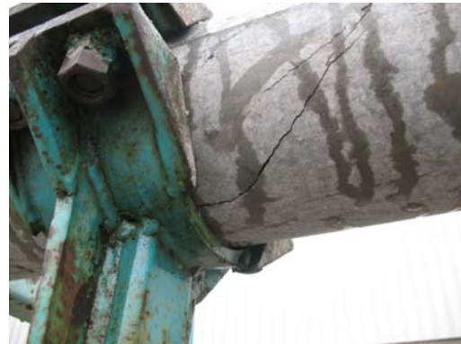
d) Cracking Pattern (collar bottom)
