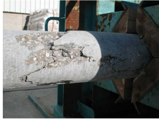
b) Failure at butt (loading side)
