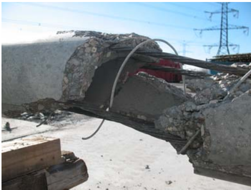
c) Failure at collar (back side)
