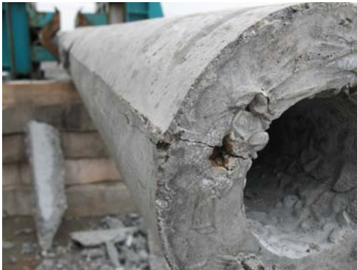
e) Strand slippage and longitudinal cracking
