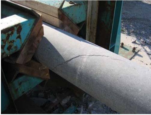
a) Initial cracking at butt
