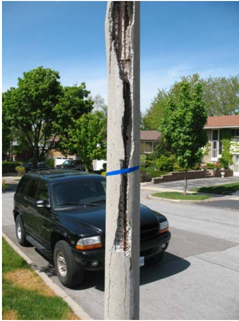
Figure 2.1: Spalling, corrosion, and longitudinal cracking of concrete pole due to segregation and differential shrinkage
