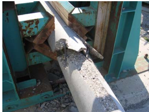
d) Failed section from above (at butt)
