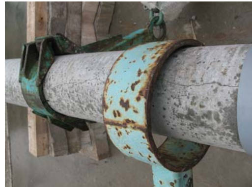
f) Longitudinal strand cracks post failure
