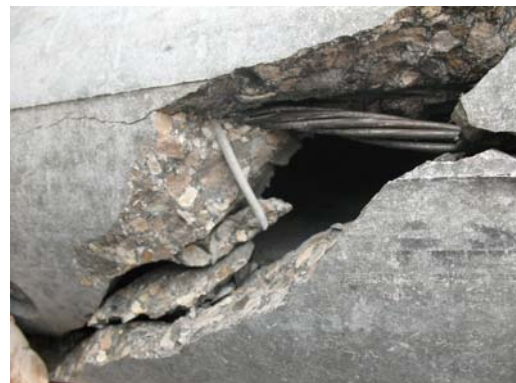
f) Crack across fail piece of helical steel
