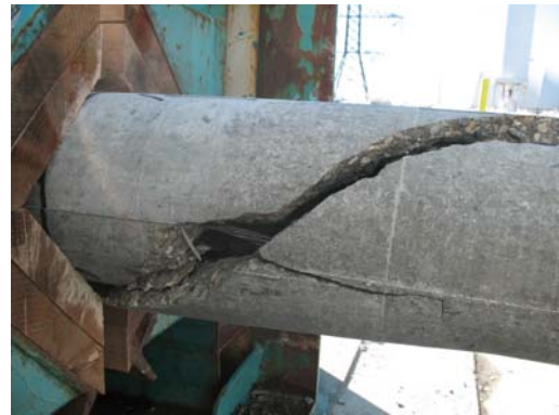
d) Failure crack on back side
