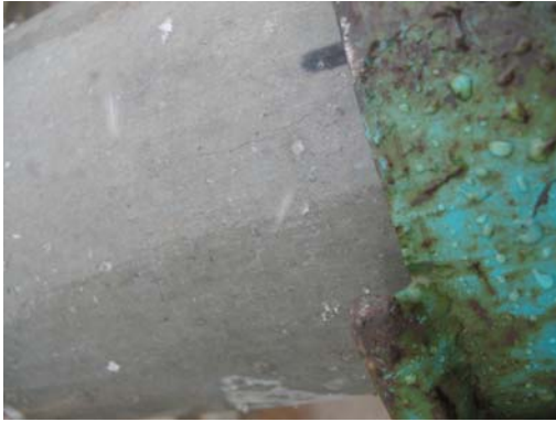
a) Longitudinal transfer crack at collar
