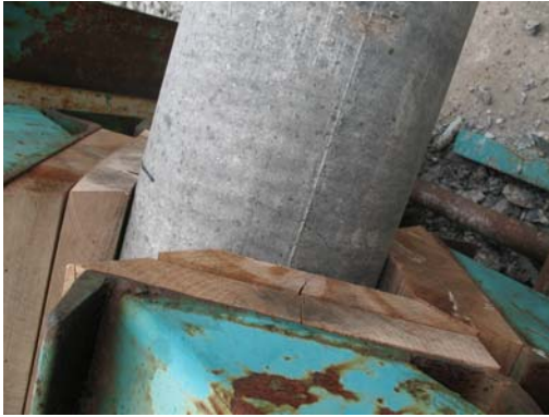
a) Initial cracking at butt
