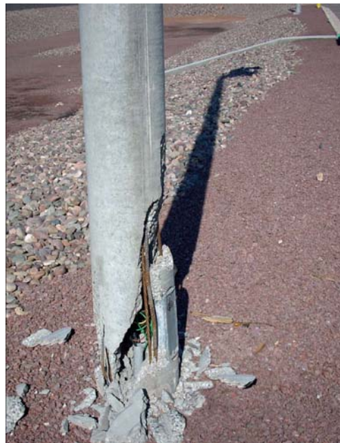
Figure 1.1: Shear failure caused by vehicle impact (Sky Cast, 2008)
