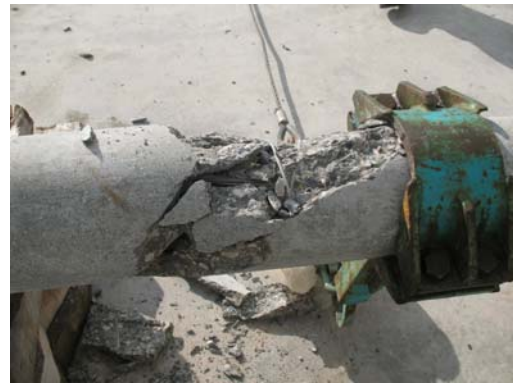
d) Failure at collar (back side)
