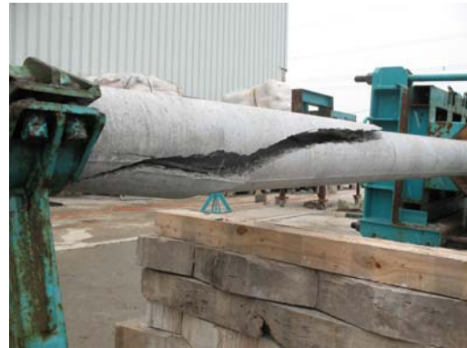
d) Cracking Pattern (front side)
