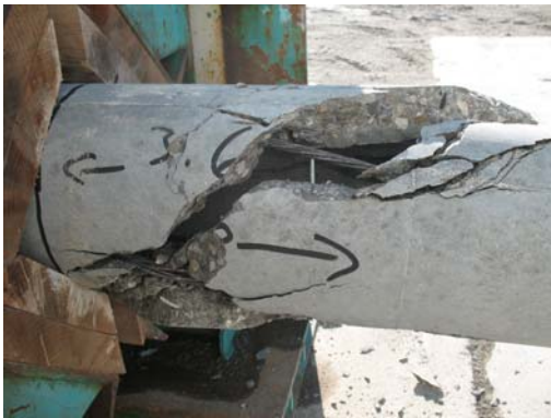
c) Failure at butt (back side). Note crack crossing failed helical steel
