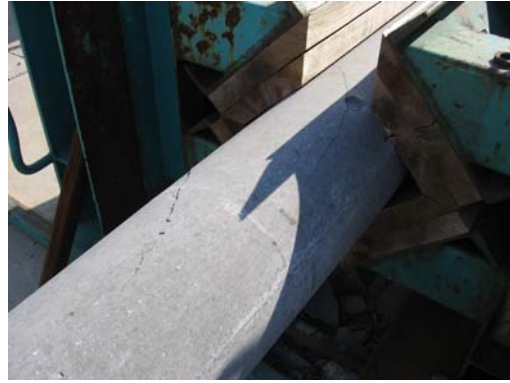
b) Torsional cracks at butt
