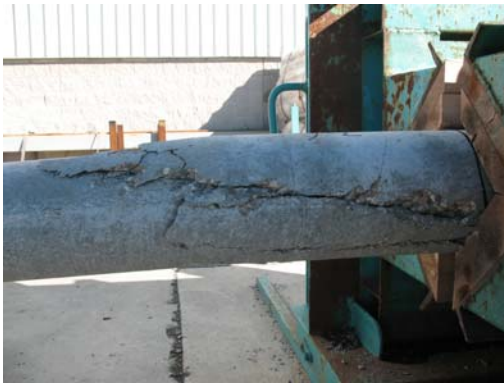
c) Crack pattern (loading side)
