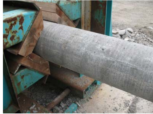
b) Two sets of torsional cracks at butt
