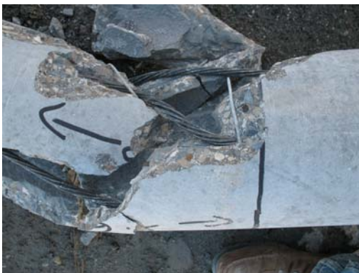
c) Failed section after removal
