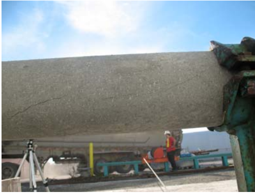
a) Torsional cracking at collar
