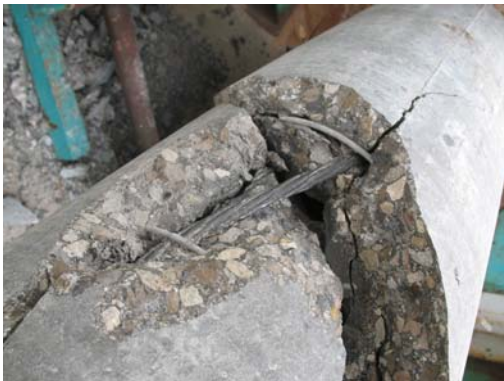
e) Close up torsional cracks crossing failed helical steel
