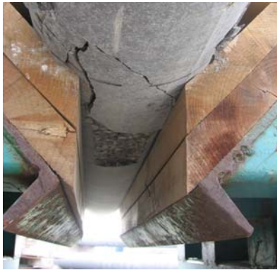
c) Cracking and spalling in butt clamp
