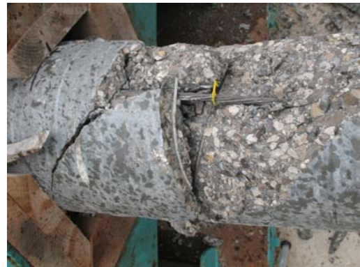
d) Failed section and cracking crossing helical steel
