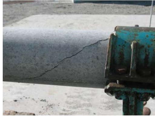
b) Cracking at collar (back side)
