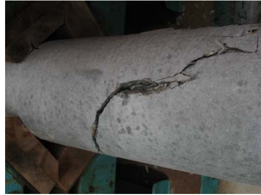
b) Torsional/longitudinal cracking at strand
