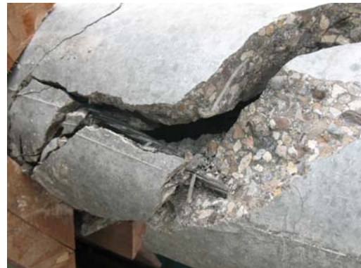
f) Torsional cracks running along helical steel and failed helical piece
