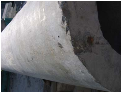
e) Longitudinal cracking at strand
