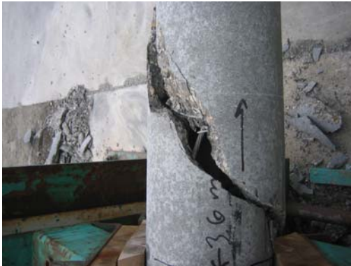
e) Failed section (from top)
