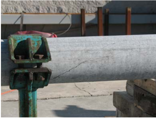
a) Cracking at collar (loading side)
