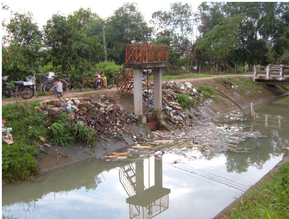
Figure 5.1 Solid waste in the concrete lined canal, TPT
