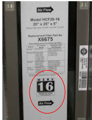
Figure 25 - Prototype House MERV 16 Air Filter
