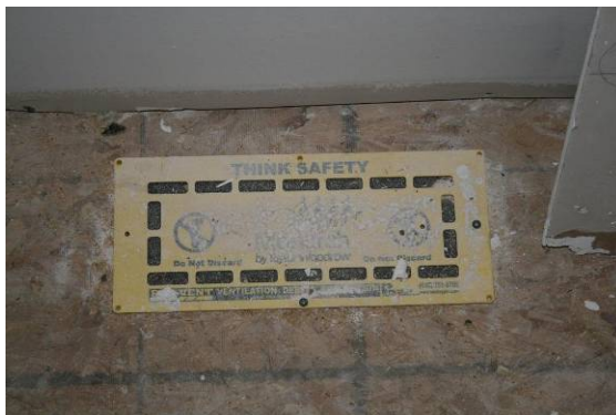
Figure 26 - Prototype House Supply Air Vent Cover
