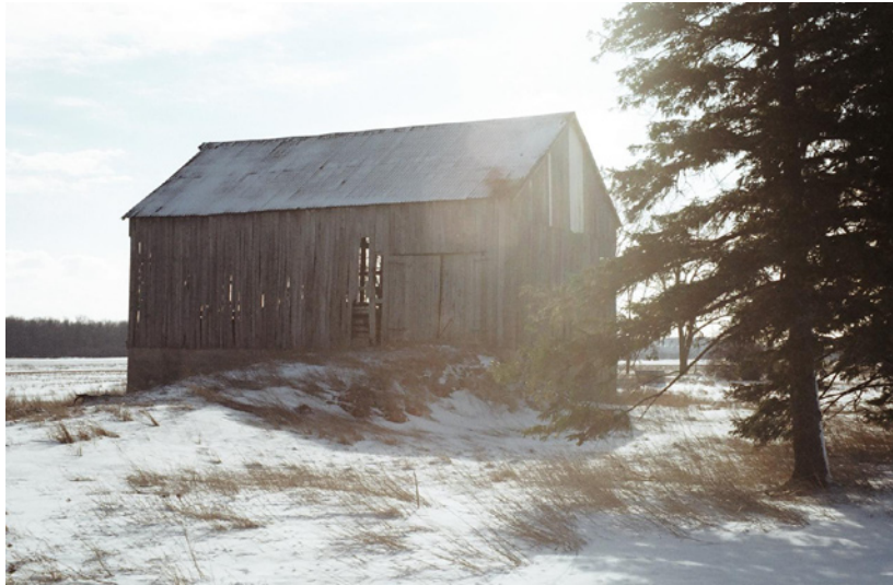
Fig5.1: Abandoned bank barn in Middlesex County. This is the versatile traditional barn type.
