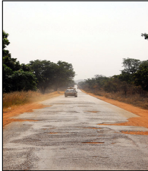
Figure 2.1: Generally, paved roads in Africa are poorly maintained creating a fragmented system with significant potholing, shoulder deterioration and unsafe driving conditions.
