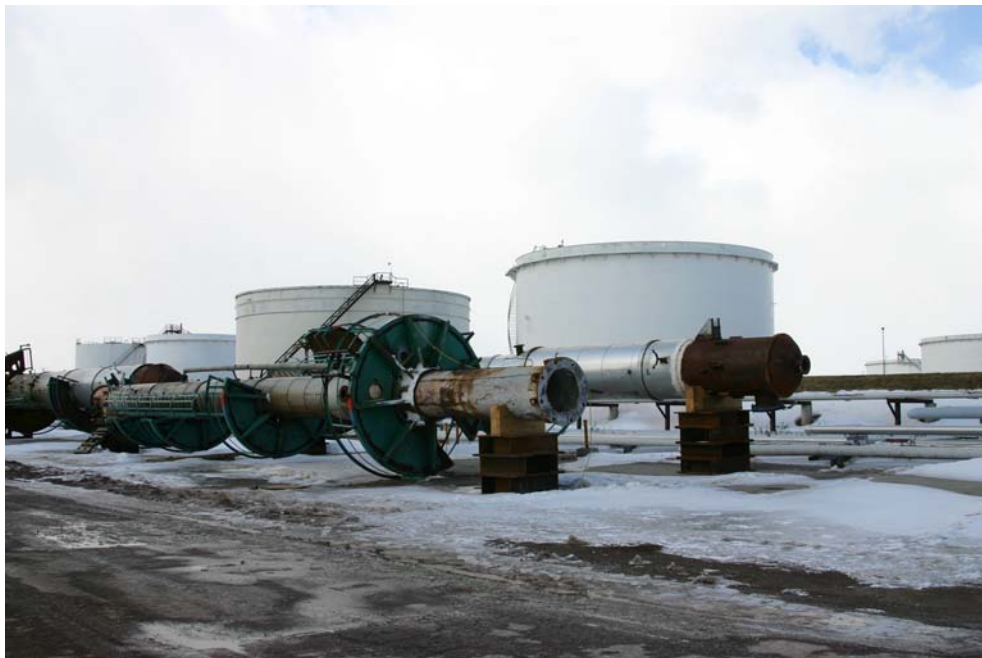
Figure 3-8: An aged “cat-cracker” is shown after its disassembly. Following the 2003 closure of the refinery, this refining equipment was no longer needed by Petro-Canada and was removed from the site.
