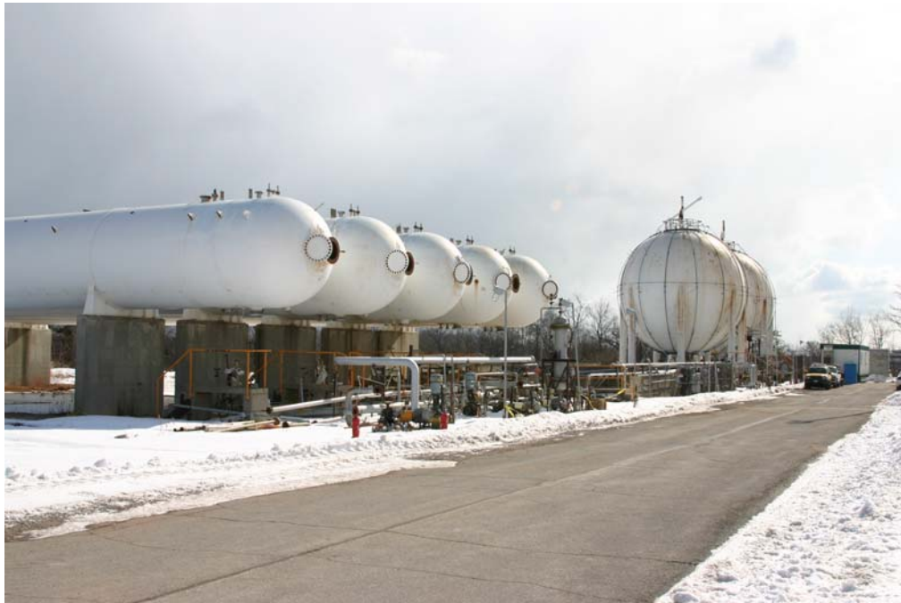
Figure 3-11: Propane and Butane tanks are slightly smaller than gasoline tanks and there are only six in total in the entire site.
