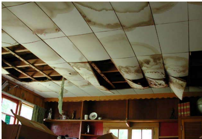
Figure 2-15: A residence built in the post war period shows signs of mould around both the exterior and interior of the building. The hollow structure was poorly insulated and sealed, causing water leakage that led to mould. Though it was cheap to build, it now faces very expensive repair costs and requires a large amount of energy to heat and cool.
