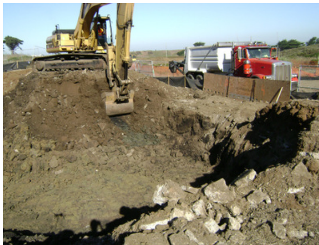
Figure 2-12: The common “Dig and Dump” procedure involves taking contaminated soil out of the ground and trucking it to a landfill. Though this procedure allows for immediate development on a contaminated site once all the toxic soil is removed, it really only lays a new problem for landfill workers. This is also an extremely costly solution, usually costing millions of dollars in large industrial sites for merely removing the soil. However, if the development of the site means better infrastructure and economic development, accommodating the surrounding area in an efficient manner, then it can be worth paying the big bucks.
