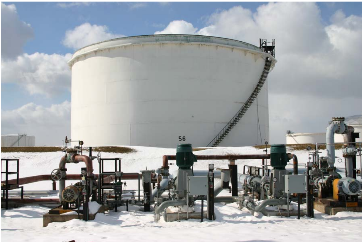
Figure 3-9: An average gasoline tank in the Petro-Canada Refinery measures an astonishing 114 feet in diameter (approx. the width of a football field) and 60 feet high (approx. 6 storeys). In February of 2002, there were 42 tanks spread across the Petro-Canada Site.
