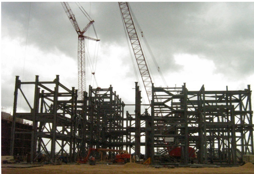
Figure 3.1 – Sandow Steam Electric Station (June 2007) (Photo Credits: S. N. Razavi)
