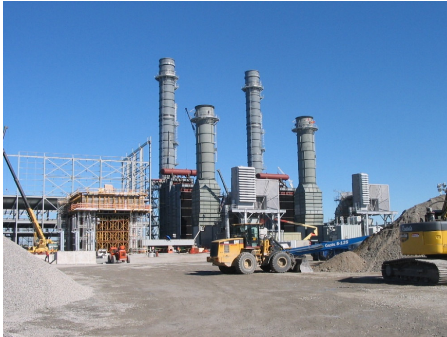
Figure 3.2 – Portlands Energy Center (November 2007)
