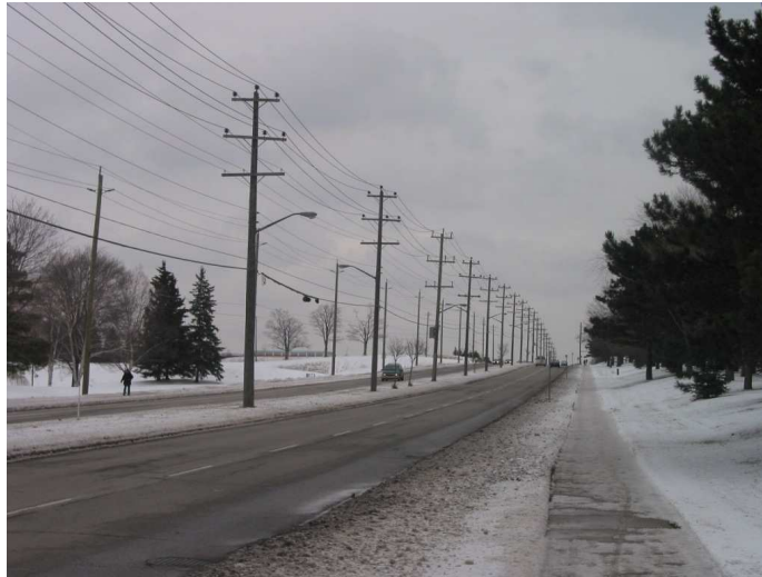
(b) 44 kV distribution line
