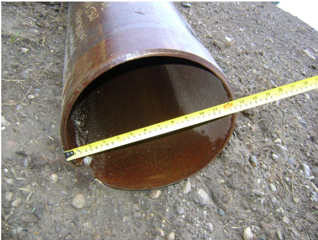
Figure 3-17: Steel Conduit Used for Cable Crossing
