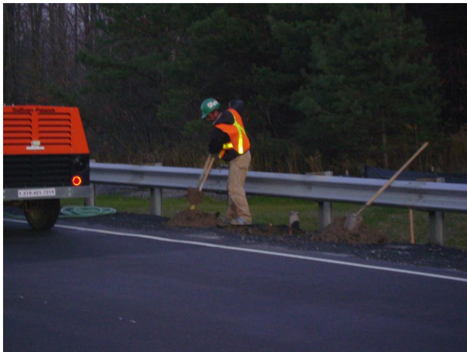
Figure 3-30: Conduit end on the Highway Shoulder and the Box where Cables are protected
