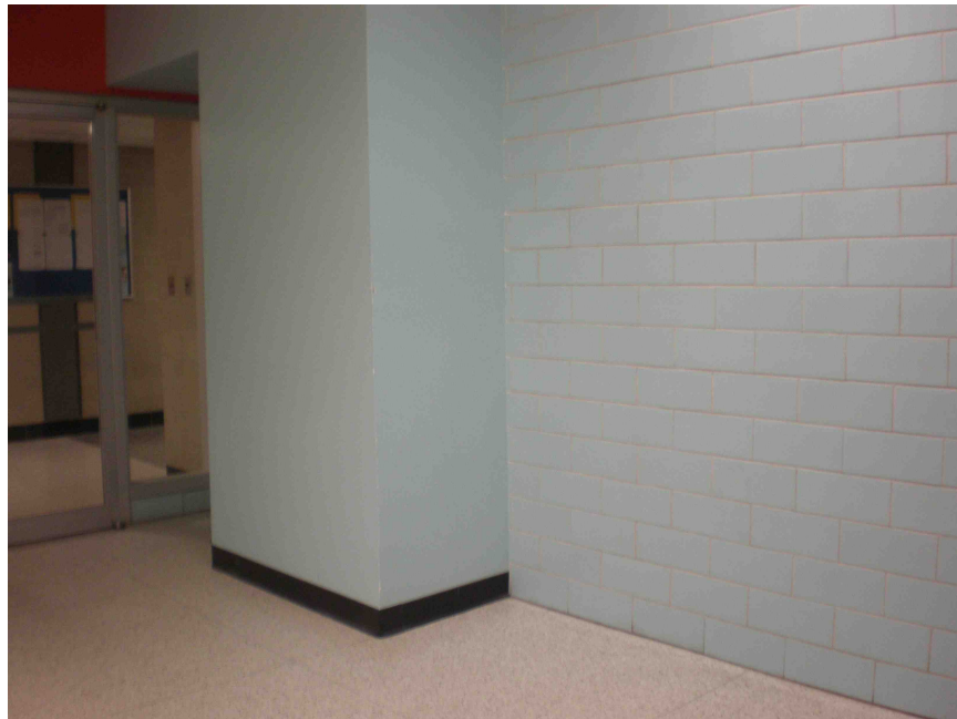
Figure B.1: Photograph of the FD2 location. The wall to the right of the picture was measured. Notice the section of wall extending into the measurement area.
