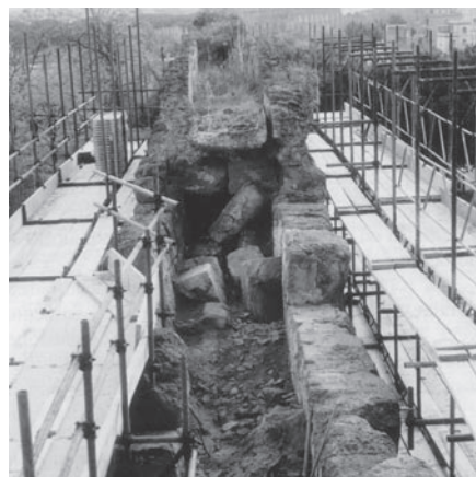
fig.4.45 ACCUMULATED DEBRIS ALONG THE AQUEDUCT CONDUIT - (BEFORE RESTORATION)
