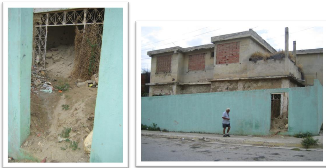
Figure 19: Housing still buried in 2008 after debris flows of 1999
